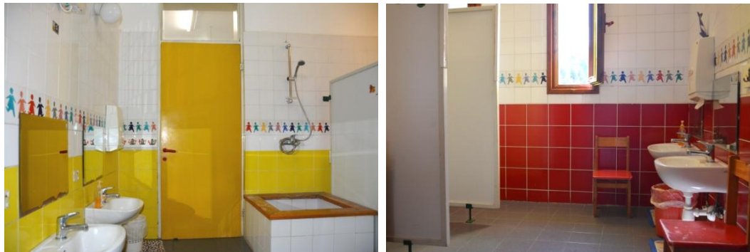
Figure 55: Shared bathroom between two classes, contains shower, toilet and lavatory - S.O.S Kindergarten (Direct Observation on 22/02/2016)
