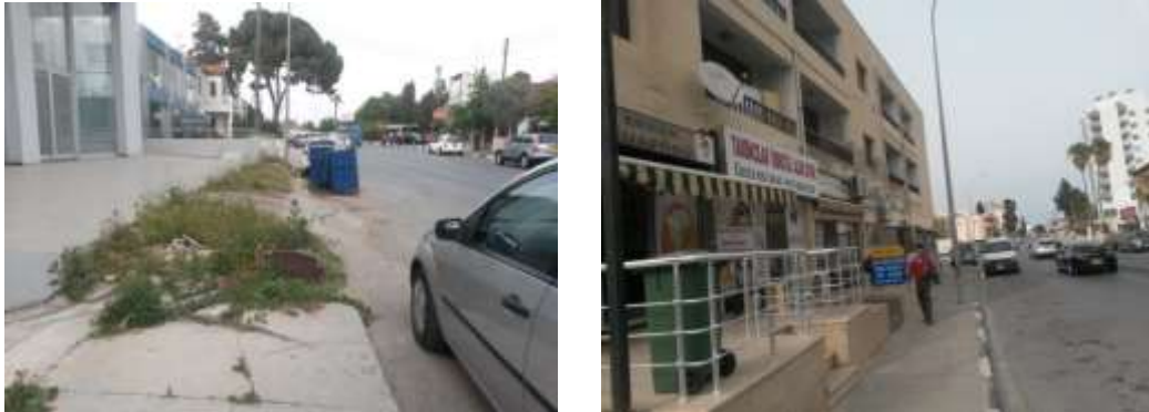
Figure 48: Poor quality of pavements and height variations in sidewalks
