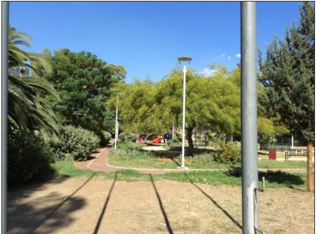
Figure 3.53: Unmaintained greeneries and defective lighting elements
