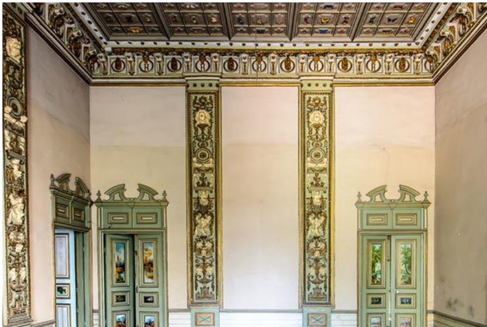
Figure 50. Interior decoration of Mostufiolmamalek house belong to the second period of Qajar (URL 28).
