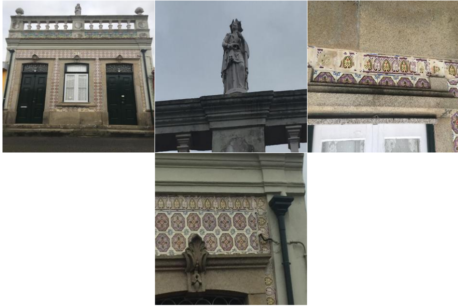
Figure 5.55: The preservation of building No 48, R.Marechal Zagalo, Ovar Photo by Shahrbanoo Dec, 2016
