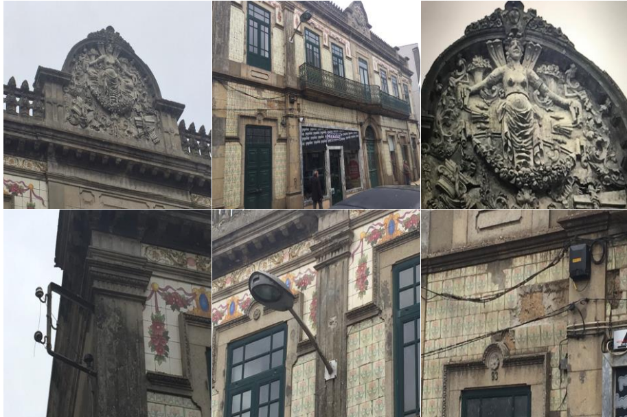
Figure 5.57: The preservation of building No 50, R.Elias Garcia, Ovar Photo by Shahrbanoo Dec, 2016
