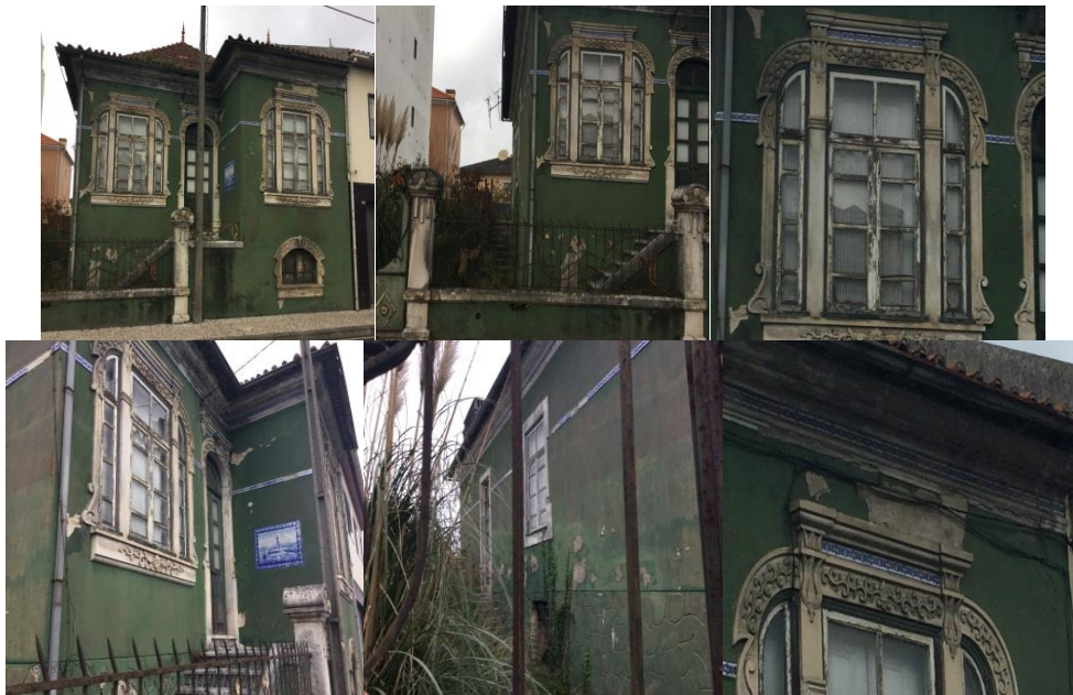
Figure 5.40: The preservation of building No 35, Rvasco da Gama Photo by Shahrbanoo Nov, 2017
