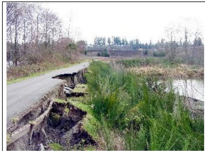
Figure 3.2: The Observation of Lateral Spread Failure after Nisqually Earthquake in Olympia, Capitol Interpretive Center (2001).
