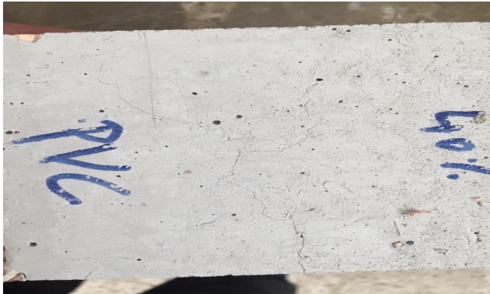
Figure 4.12: Presence of Surface Cracks
