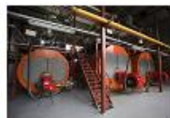
Boilers & Process Heat
