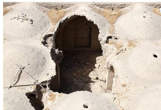
Figure 83. Deterioration in the roof of warehouses
