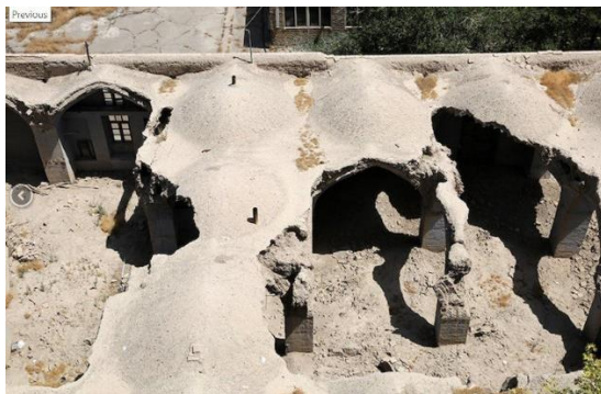
Figure 82. Deterioration in the roof of warehouses
