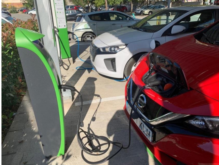
Figure 2.15: Electronic Car Charging System
