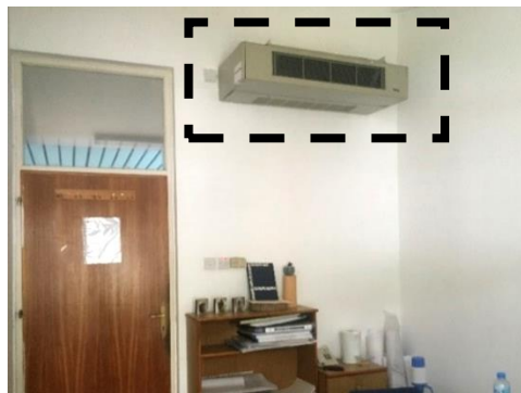
Figure 54: Typical Mechanical Cooling&Heating Unit in an Office Room (Taken by author, 2018)
