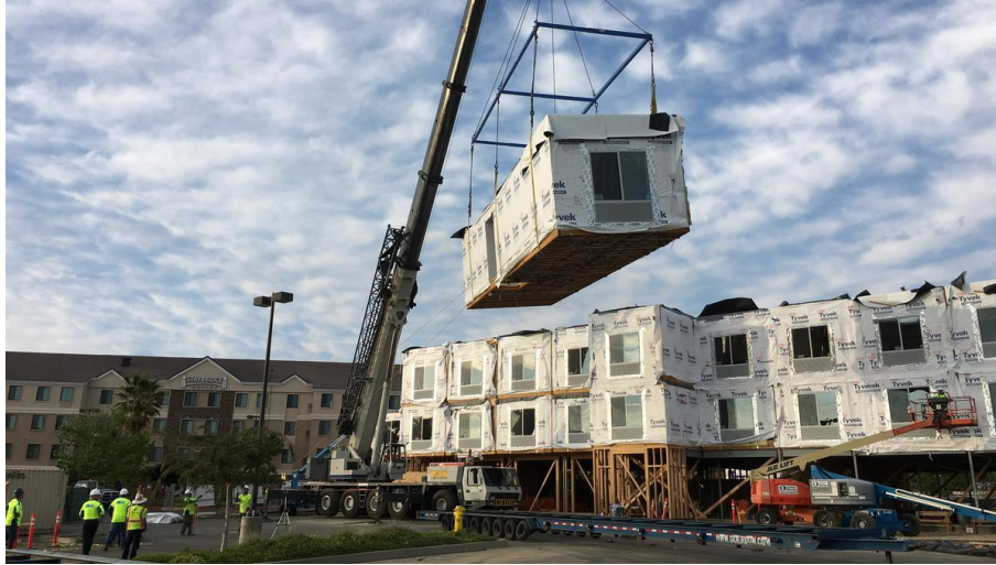
Figure 44: Fairfield Inn & Suites hotel modules being installed in the site, Folsom, California (URL39)
