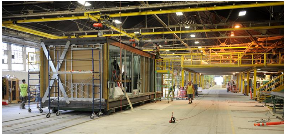
Figure 43: Modules being assembled in the factory DeLuxe Building Systems, Berwick, PA (URL38)
