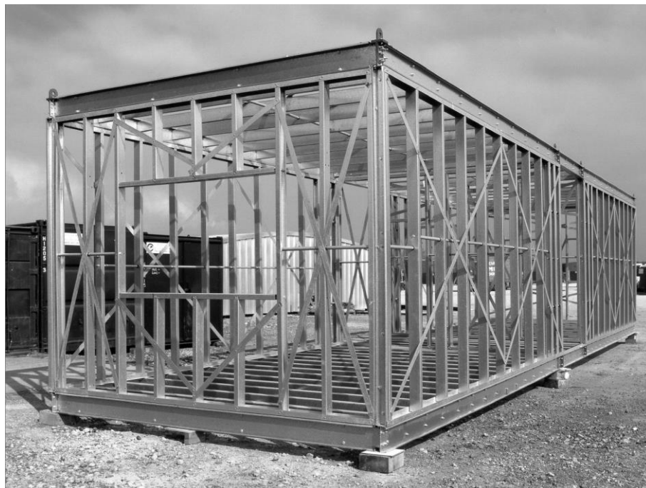
Figure 38: Illustration of a modular unit that is edge-sustained with a middle corridor. (URL42)
