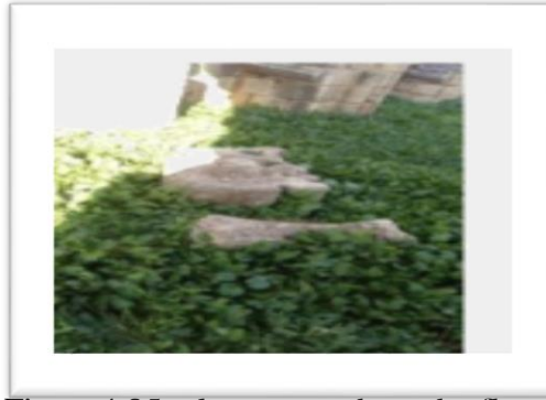
Figure 4.25: plants growth on the floor
