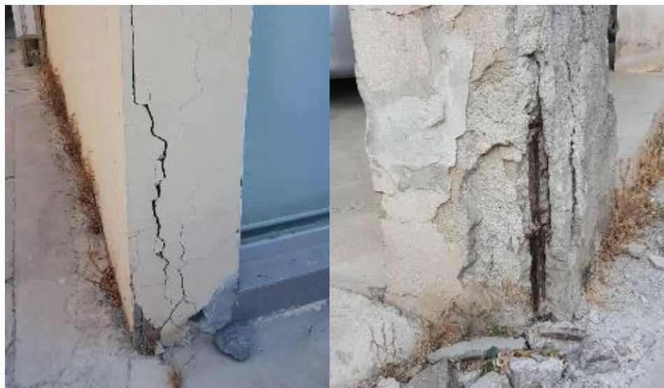
Figure 1.1. Longitudinal cracks due to corrosion deterioration in a column.
