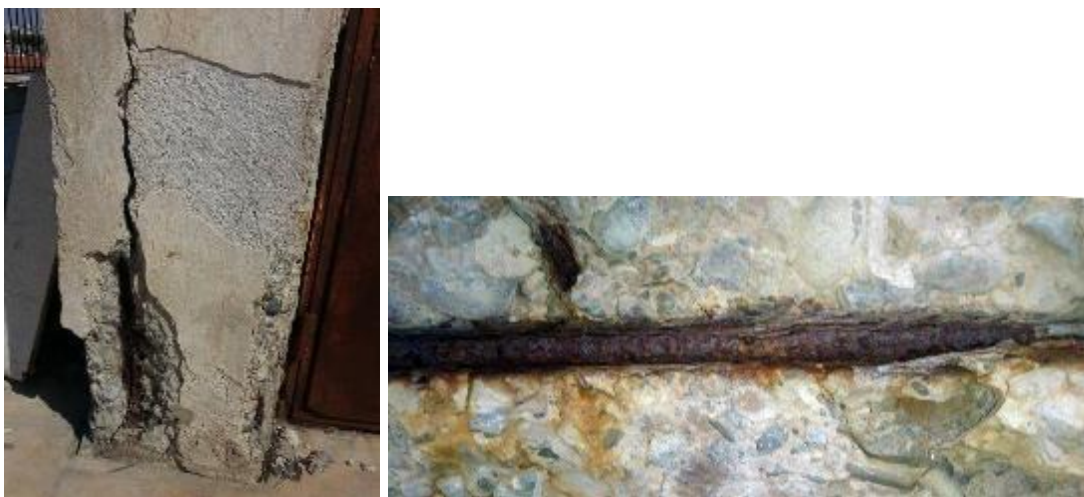
Figure 2.1. Corrosion deterioration on reinforced concrete elements
