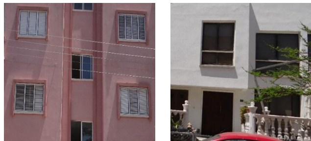
4.57: Frame windows material, Famagusta (author).
