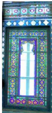
Figure 3.11: Window of an Iranian traditional house in Kashan, Iran; (Iran / Iranian Historical Photographs Gallery, 2010; kashan 29).
