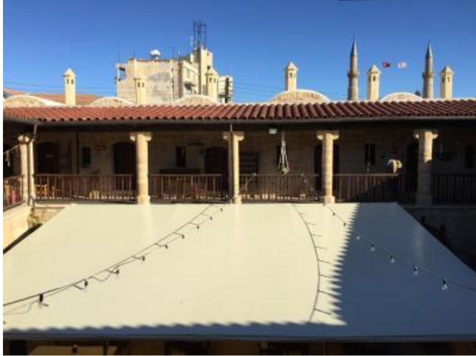
Figure 3.35: Lighting system after the conservation of the Kumarcılar Hanı. (Author, 2017)
