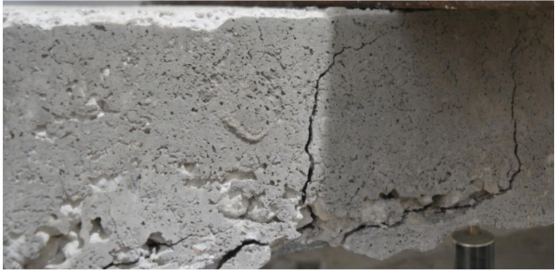
Figure 4.20: Longitudinal shear failure mode for specimen mk-LS1s.
