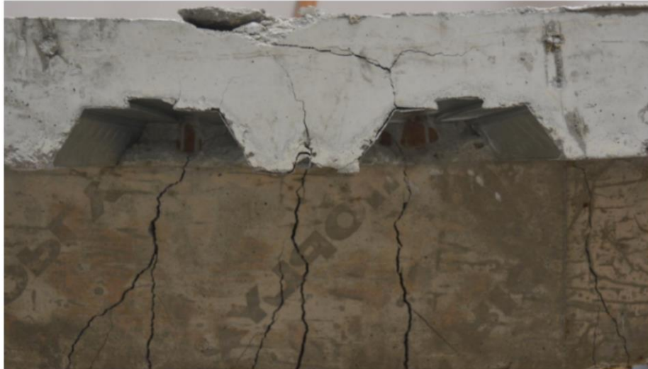
Figure 4.2: Cracks on the reinforced concrete beam after failure of specimen CS.
