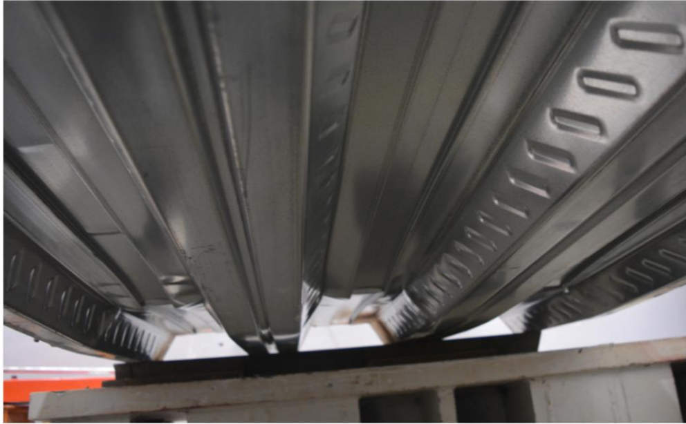
Figure 4.12: Buckling failure of the steel sheet web.
