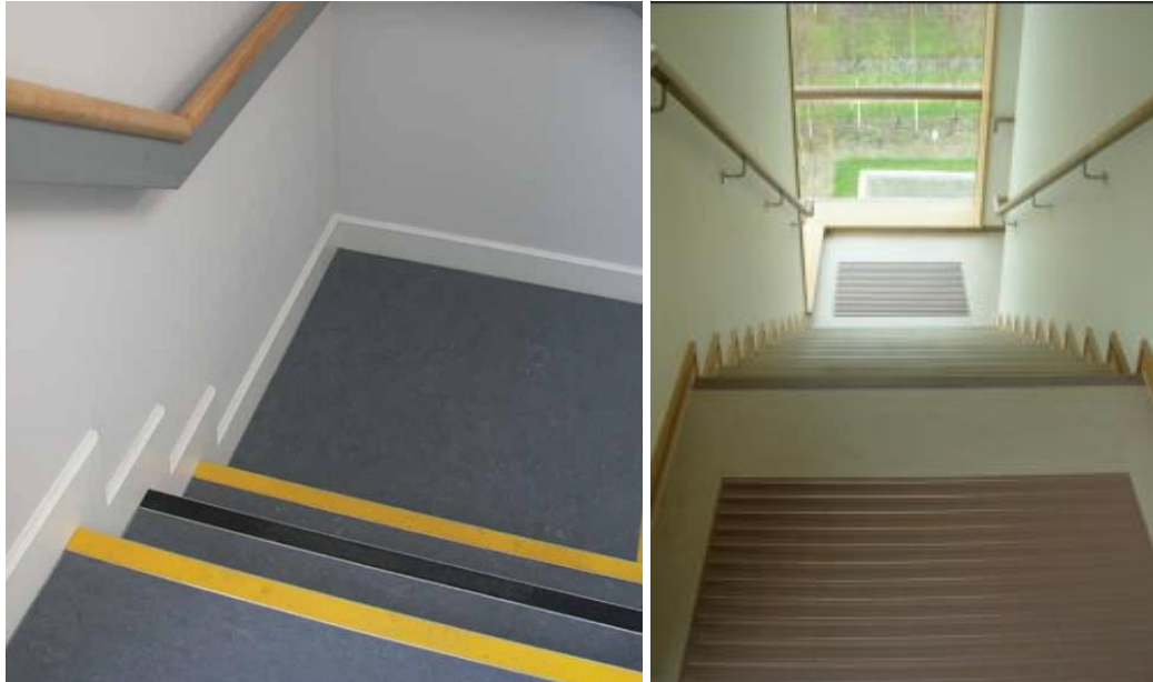
Figure 12: Examples of staircase with non-slip applied nosing and tactile surface at top and bottom of steps (retrieved from http://universaldesign.ie )
