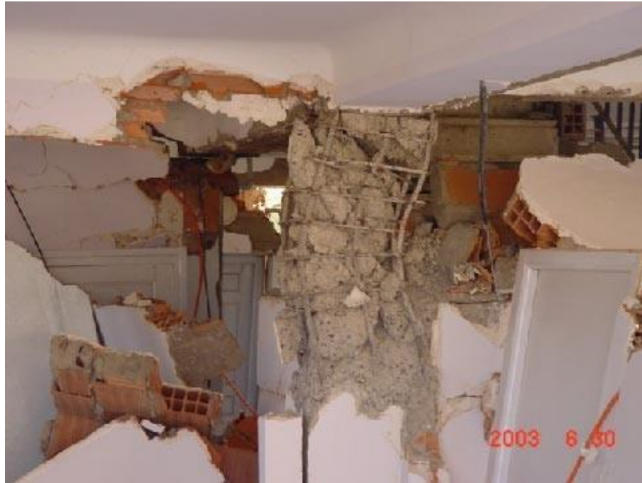
Figure 2.1: Staircase column damage Zem-mouri earthquake in Algeria (Bechtoula & Ousalem, 2005).
