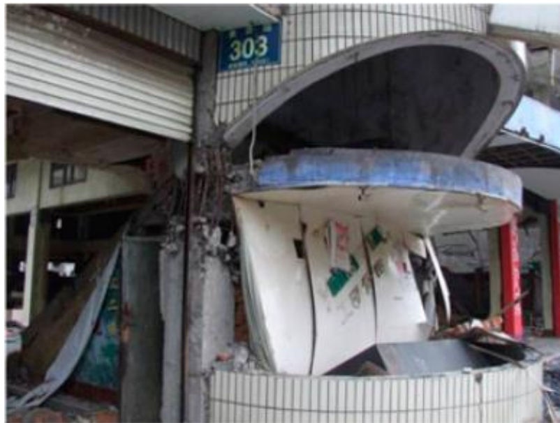
Figure 2.3: Beam-column connection damage Wenchuan earthquake China 2008 (Li & Mosalam, 2012).
