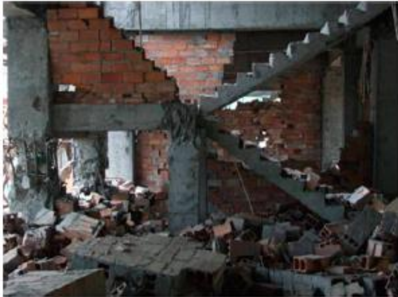
Figure 2.2: Short column damage Wenchuan earthquake China 2008 (Li & Mosalam, 2012).
