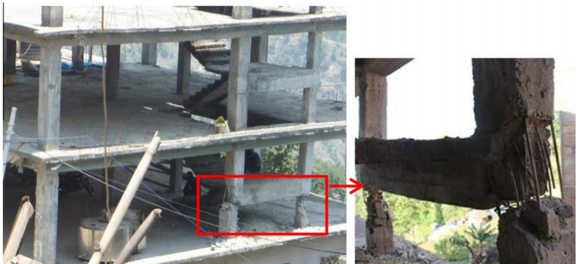
Figure 2.4: Short column failures Gorkha District of Nepal on April 25, 2015 (Sharma, Deng & Noguez 2016).
