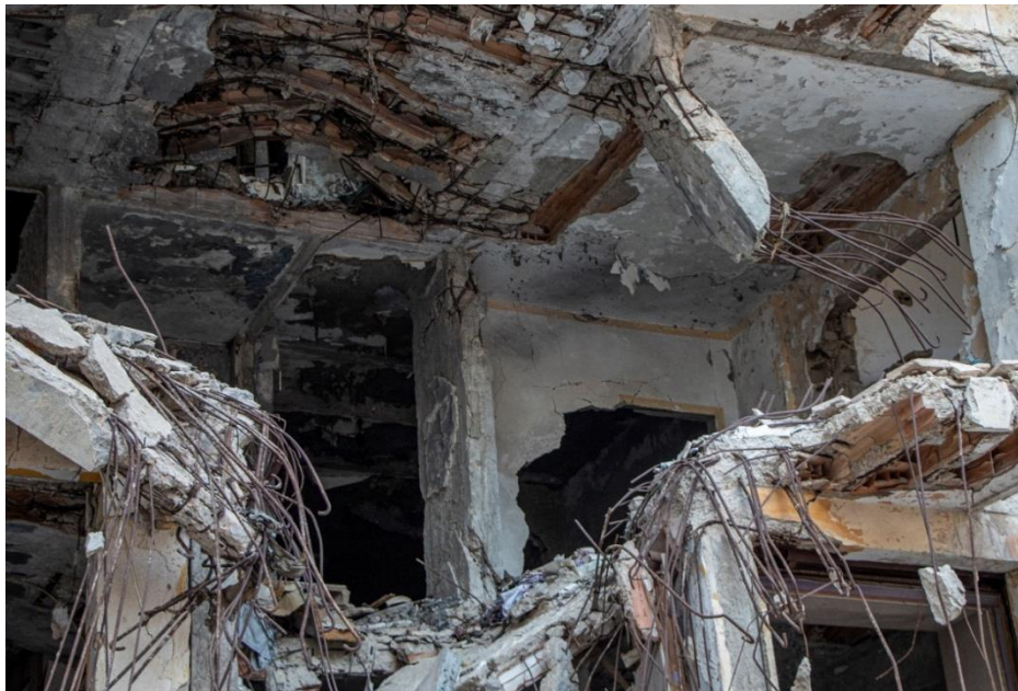
Figure 5.2: Broken Two Main Columns and Slab
