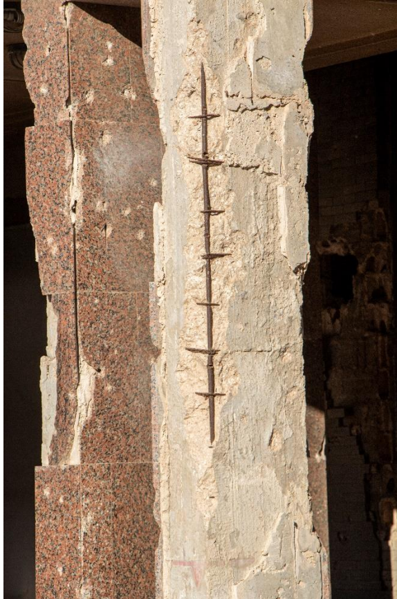
Figure 4.7: Partial Material Losing in A Column
