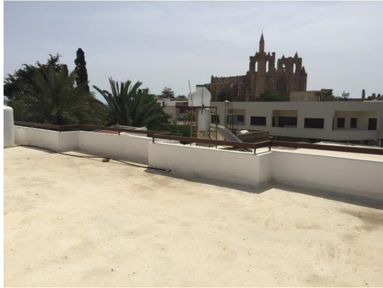
Figure 37: The roof terrace of Efecan Building Complex; (Author, 2019)
