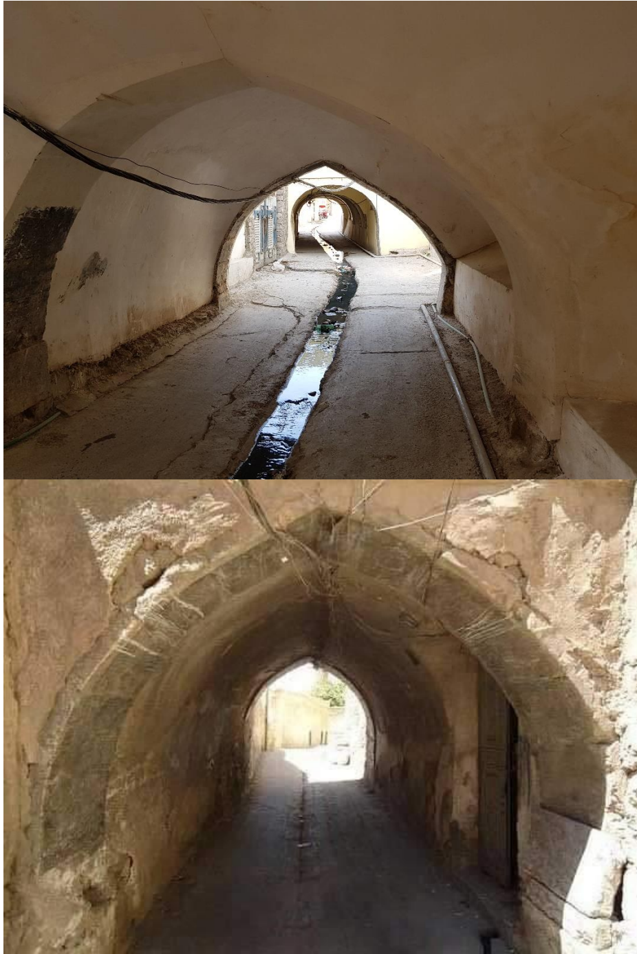
Figure 35: Qanatir in the Old City of Mosul (Archways) Source: First, Author, Second, Iraq museum
