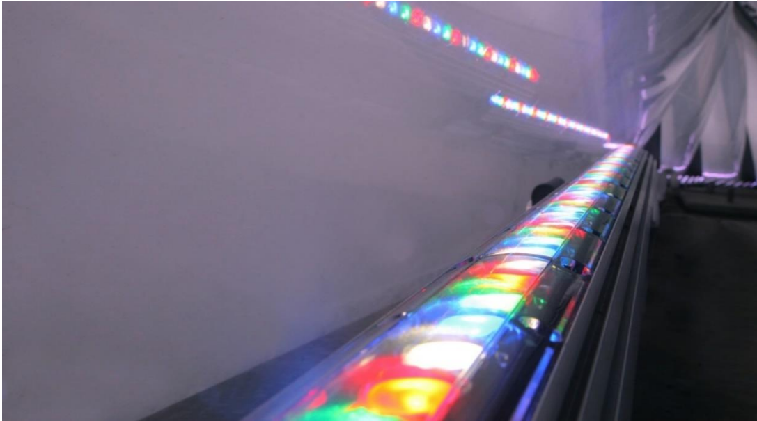
Figure 4.13: The Installed LED Lights for Allianz Arena (Lighting Philips, 2016)
