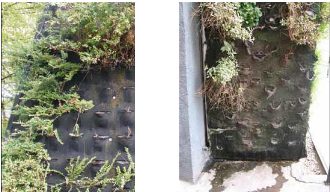
Figure 24: (a) (left) felt layer with dead plants (b) (right) substrate with tears, degrading felt layer and water leakage (Tarboush, 2019).
