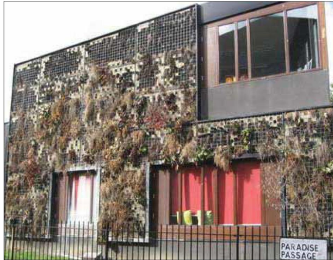
Figure 25: Living wall panels degradation, Islington, North-London (Tarboush, 2019).
