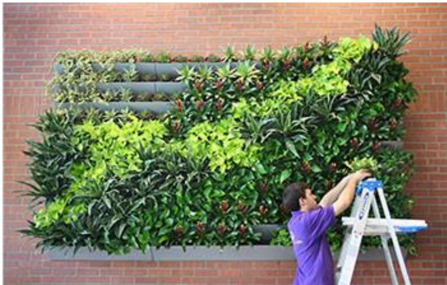
Figure 15: Example of modular trays living wall (Tarboush, 2019).
