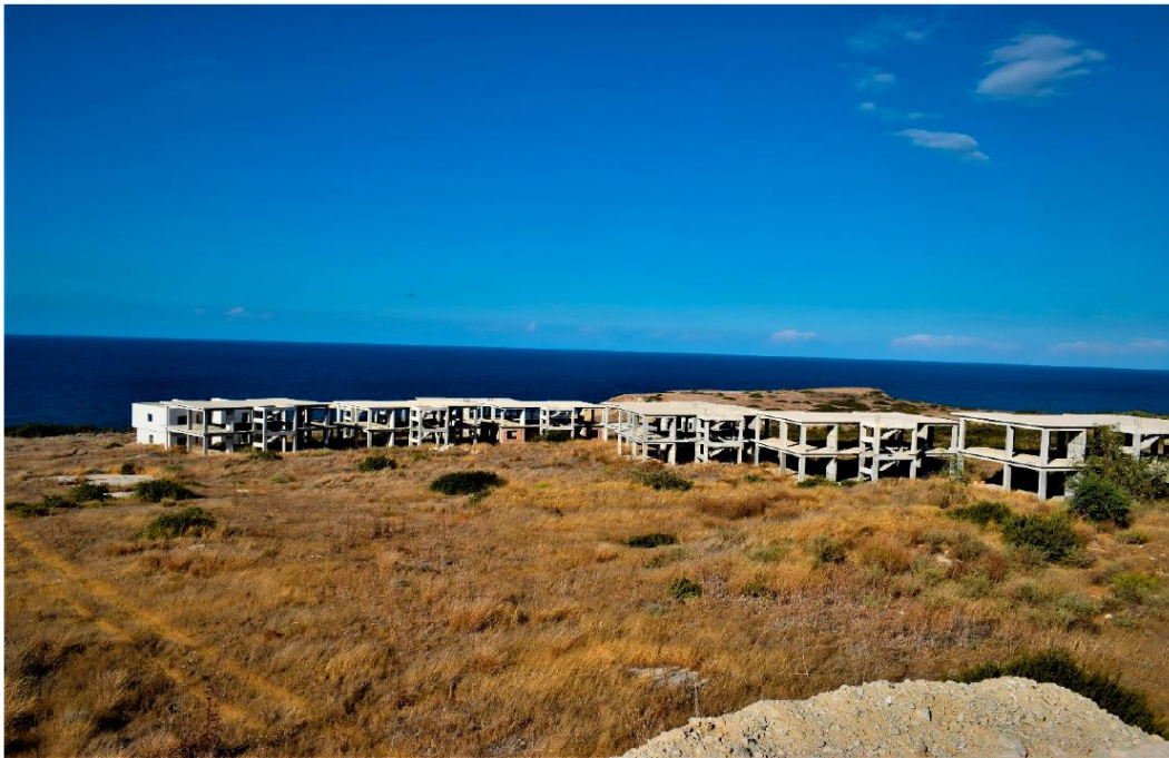
Abandoned illegal development, Tatlisu coastal zone , North Cyprus Source: by Authors, 2020
