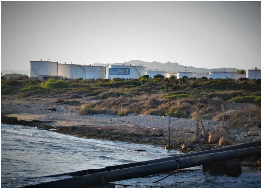
Petroleum depo. Bogaz coastal zone, North Cyprus. Incompatible location for petroleum storage. Source: by Authors,2020
