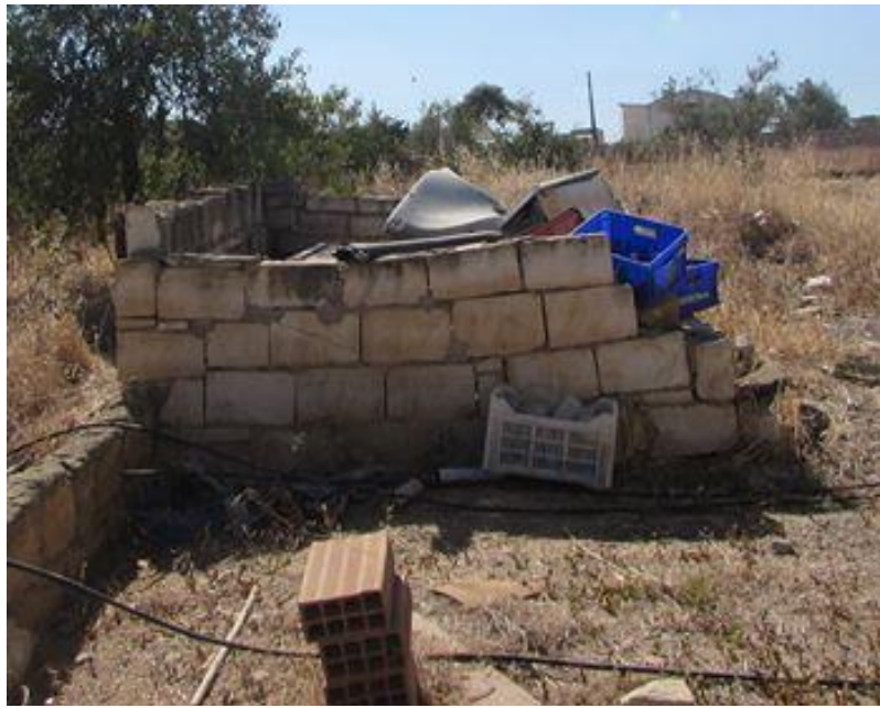
Figure 57. An example of partially demolished and abandoned external storage of traditional Cyprus houses (Author,2018)
