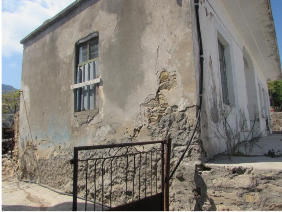
Figure 21. Example of constructed technique with stone masonry in Cyprus traditional houses (Author, 2018)
