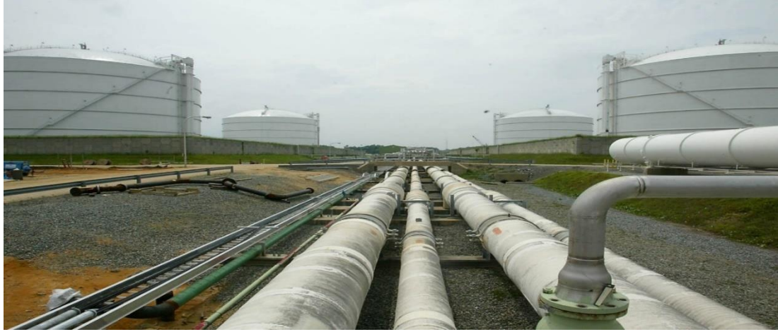
Figure 3.5: Natural Gas Pipeline
