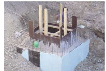
Figure 4: Worker without protective hat
