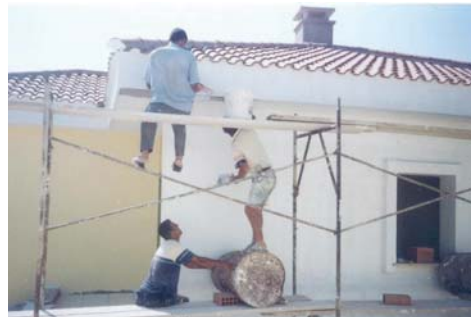
Figure 1: Unsafe scaffolding was used for external plastering and painting.
