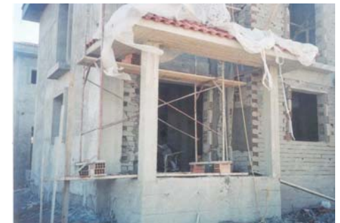
Figure 2: Unsafe scaffolding was used for external plastering and painting
