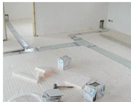
Photo 5. Detail of ventilation system. Photo taken by designer.
