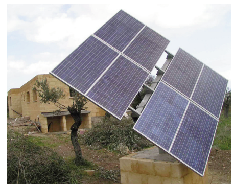
Photo 6. PV panels. Photo taken by designer
