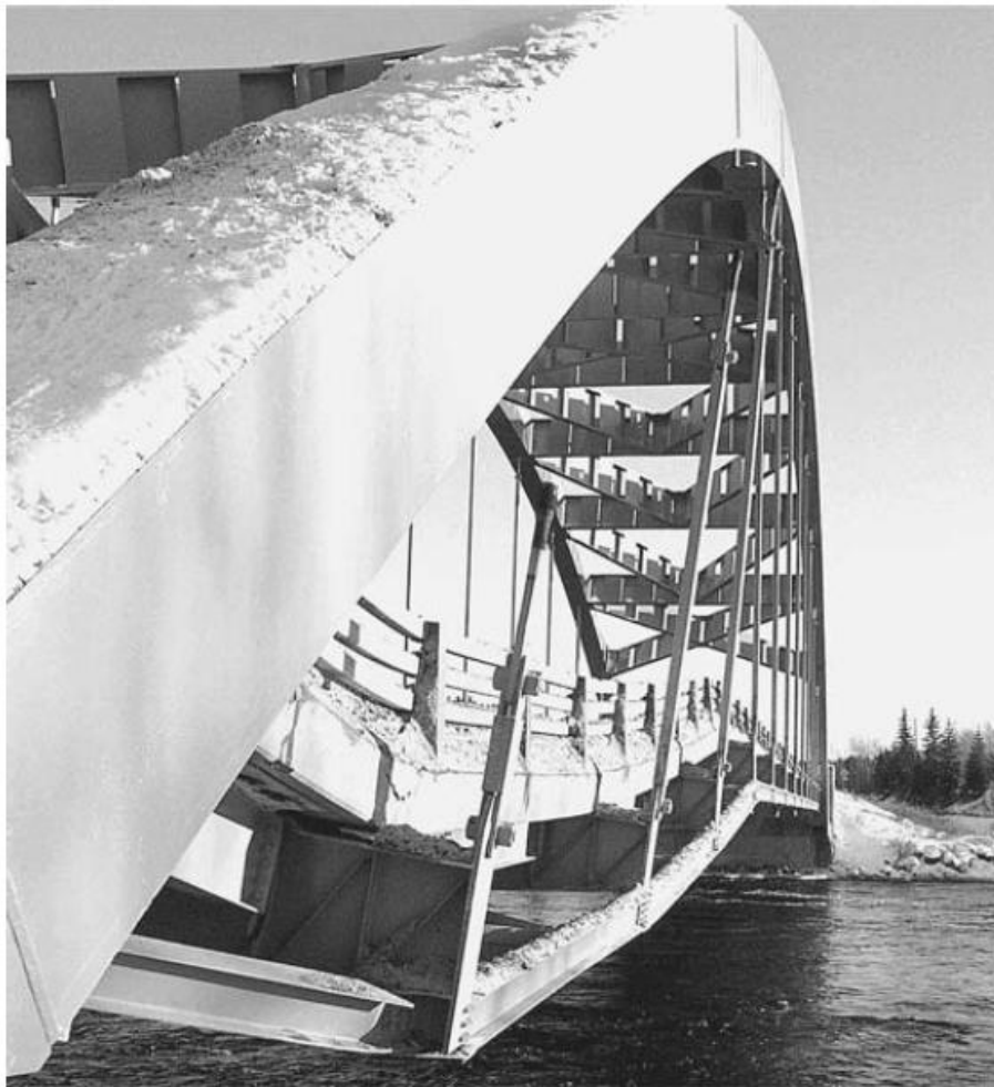
Figure 2.9: The (partial) collapse of tied-arch Bridge [15]
