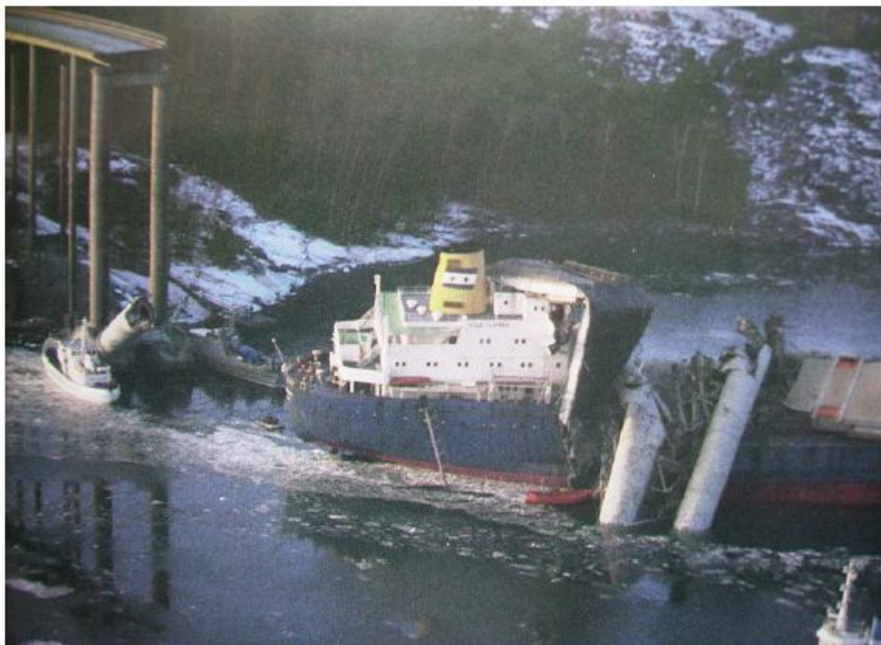
Figure 2.7: Arch bridge collapsed due to ship collision [15]
