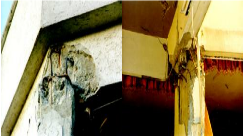
Figure 8. Beam-column junction damages.
