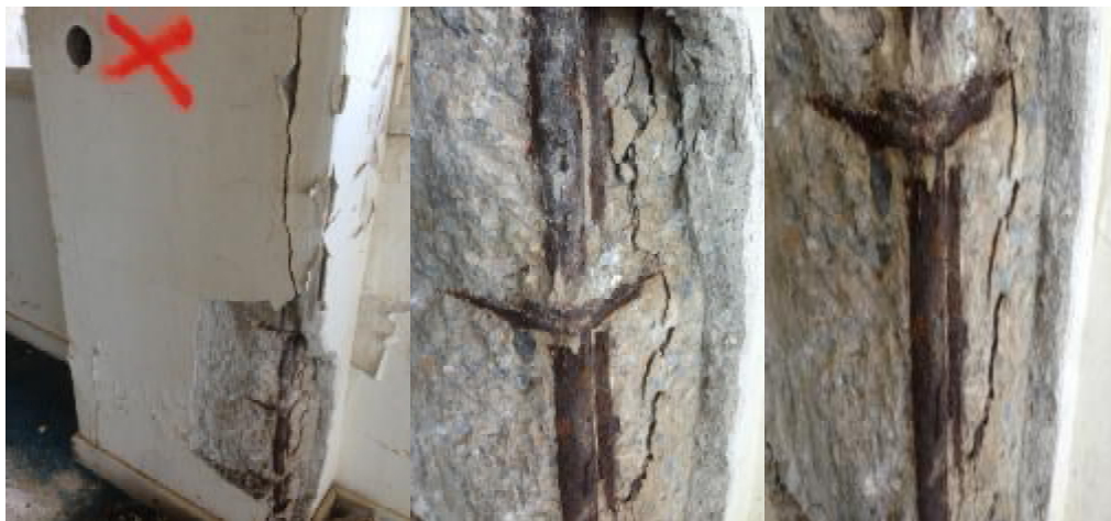
Figure 10. Reinforcement Corrosion of Column (Seaside Building).
