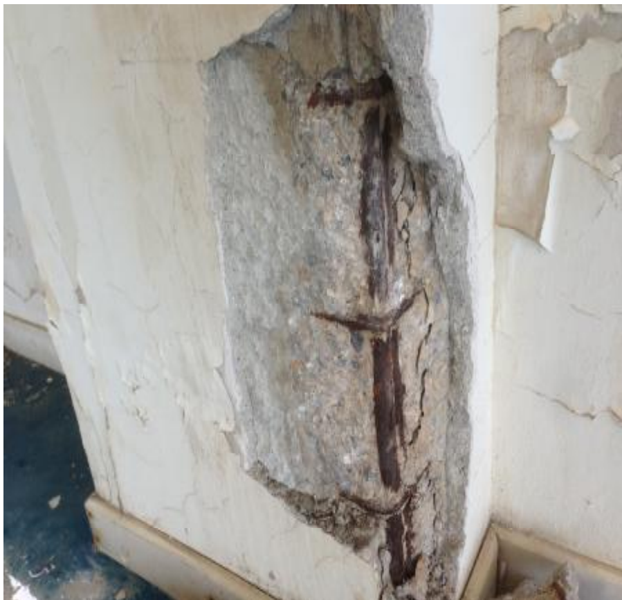
Figure 64. Corrosion problems in a column
