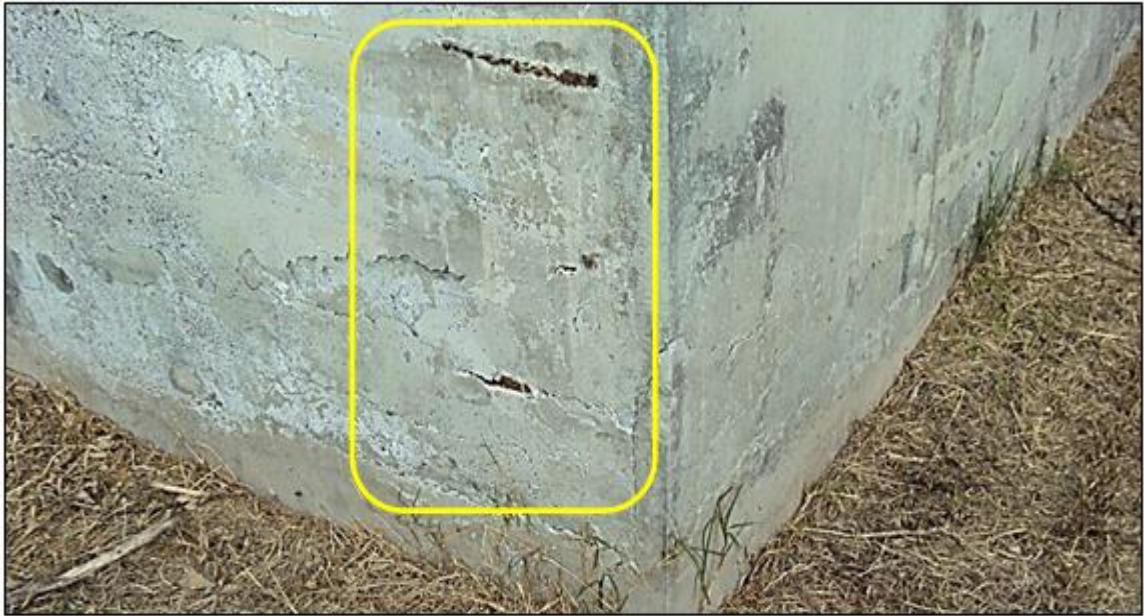
Figure 4.8: Cover Problem at the EMU Campus WWTP.
