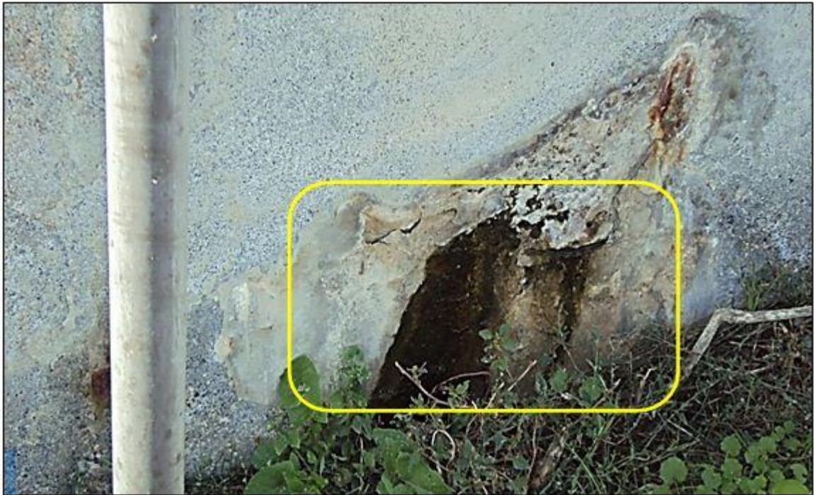
Figure 4.11: Sulphate Problem in the EMU Campus WWTP
