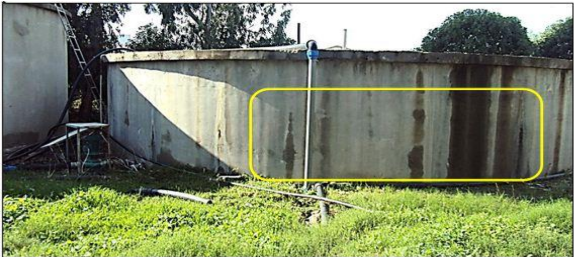
Figure 4.9: Permeability Problem at the EMU Campus WWTP.
