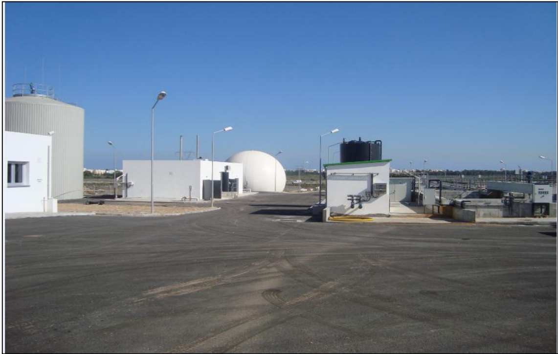
Figure 3.2: Unit Treatment Tanks of Gazimağusa WWTP
