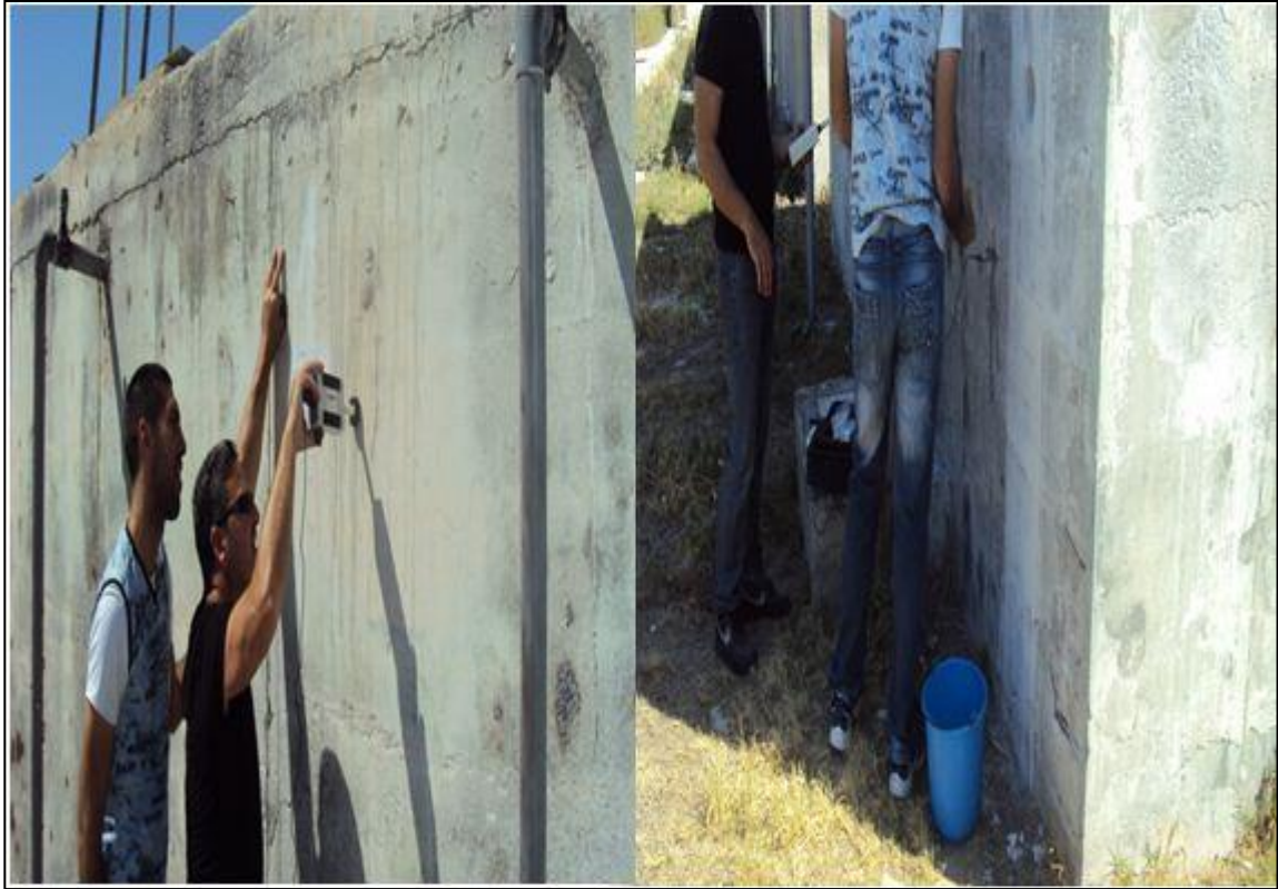
Figure 5.13: Potential Corrosion Measurement Process.
