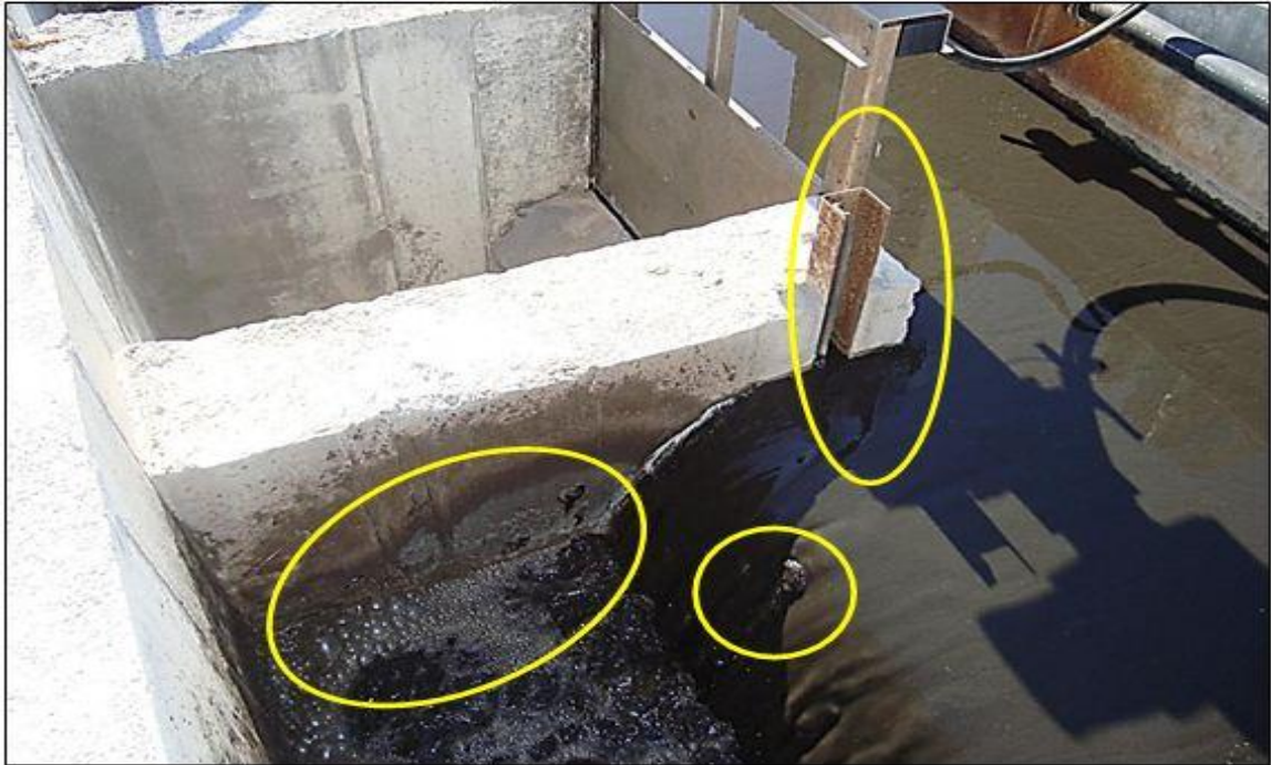
Figure 4.1: Bump Concrete and Rusting of the Steel.
