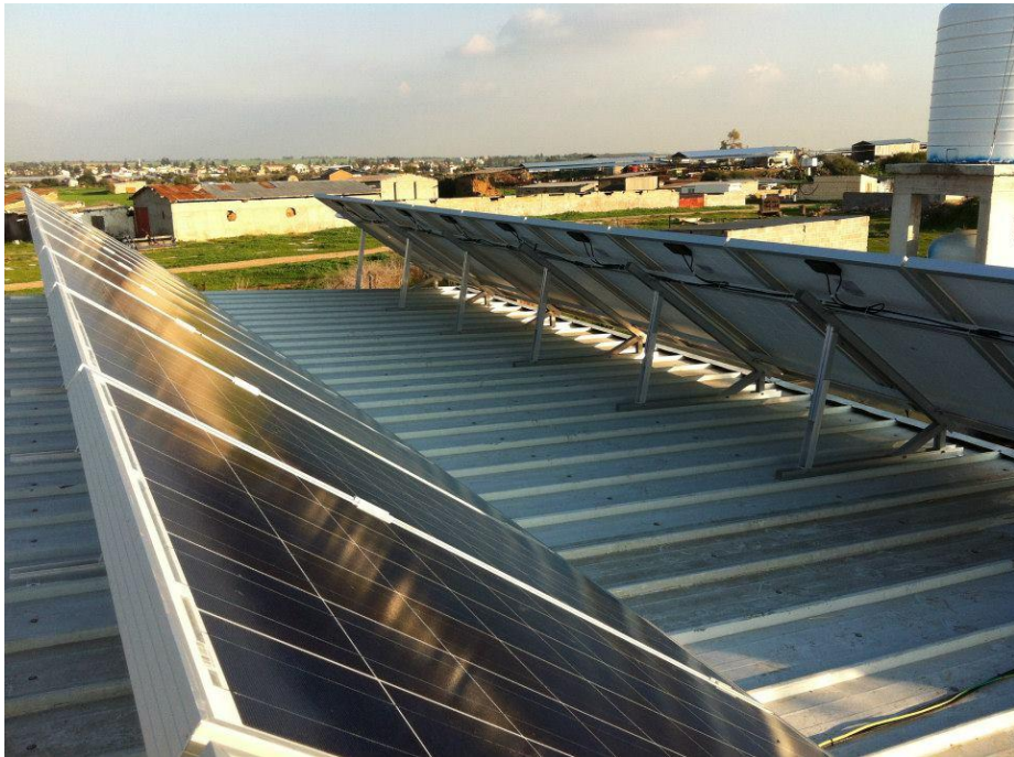
Figure 31: Cengiz Topal 5,28 kWp Off-Grid Sistem Vadili
