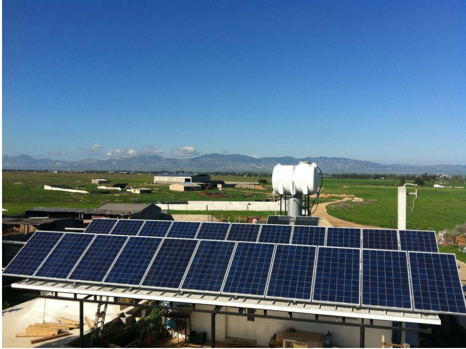
Figure 30: Cengiz Topal 5,28 kWp Off-Grid Sistem Vadili
