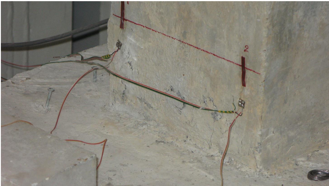
Figure 4-16: Start of crushing in compression side of column
