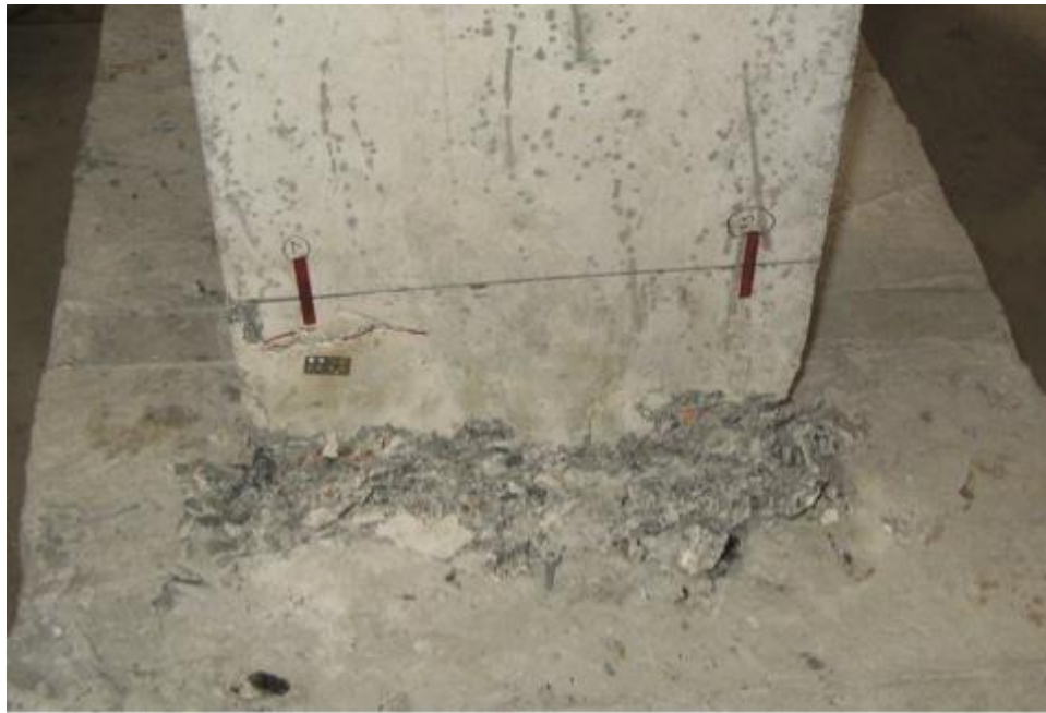
Figure 4-11: Crushing in compression side of the column with 1% fibers
