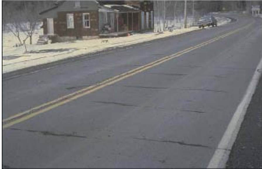
Figure 10: Low Temperature Cracking Source: (Federal Highway Administration, 2010)
