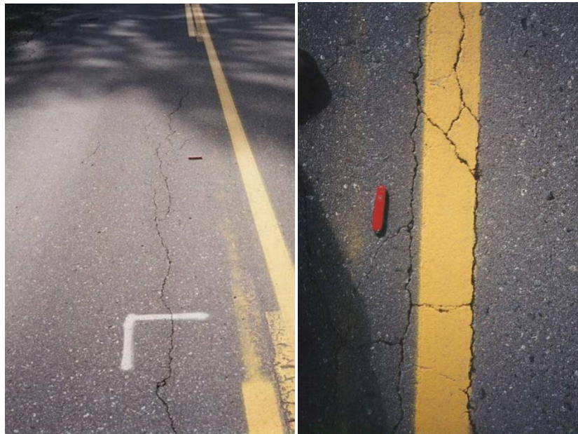
Figure 11: Low severity longitudinal cracking Source: (Opus Consultants International (Canada) Limited, 2009)
