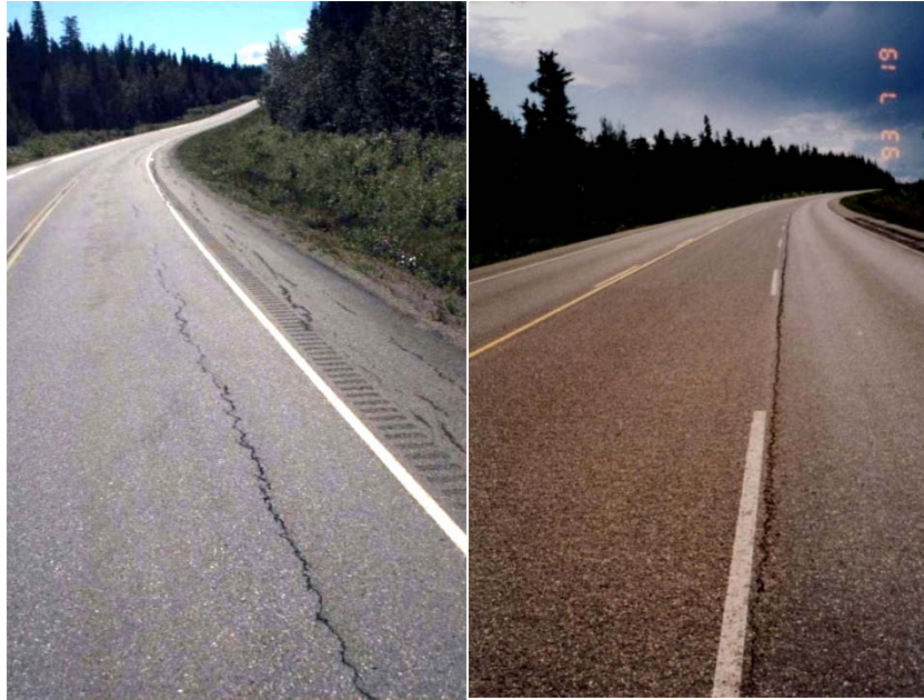
Figure 12: Medium Severity Longitudinal Cracking Source: (Opus Consultants International (Canada) Limited, 2009)
