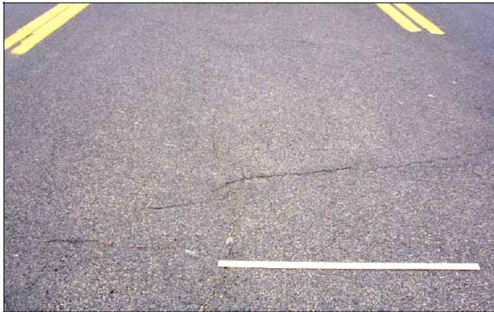
Figure 7: Low Severity Alligator Cracking Source:(Federal Highway Administration, 2006-2009)
