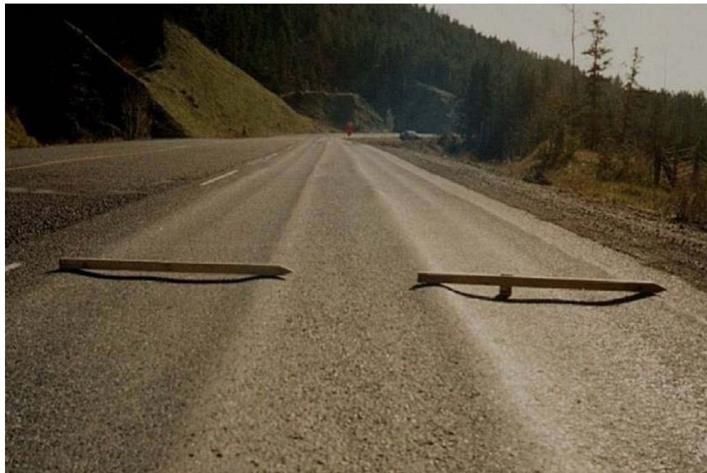
Figure 20: High Severity Rutting Source: (Opus Consultants International (Canada) Limited, 2009)
