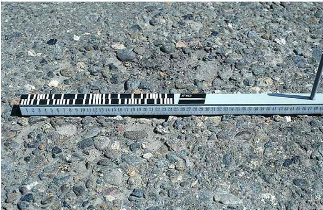
Figure 4: Loss of Coarse Aggregate Source: (Miller ; Bellinger, 2003)
