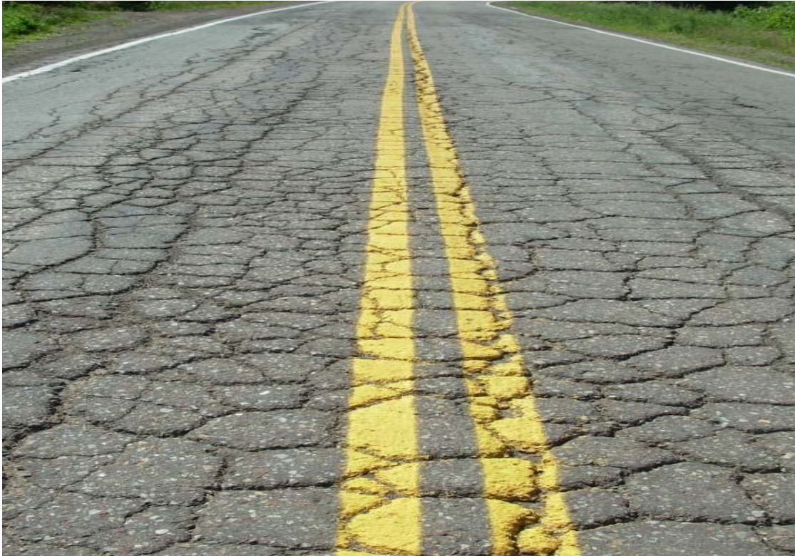
Figure 9: High Severity Alligator Cracking Source: (Opus Consultants International (Canada) Limited, 2009)
