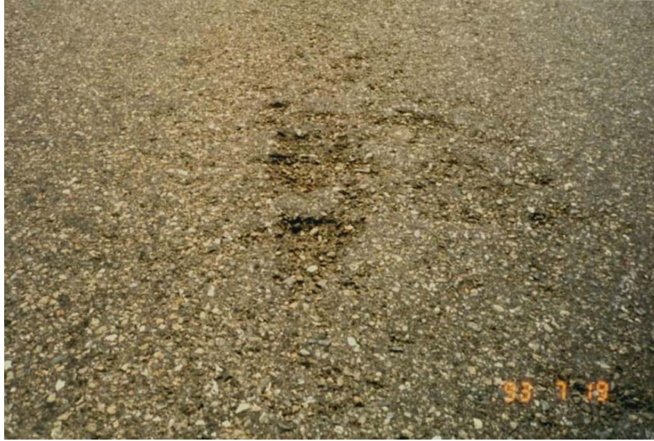
Figure 5: High Severity Raveling Source: (Miller ; Bellinger, 2003)
