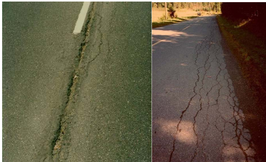
Figure 13: High Severity Longitudinal Cracking Source: (Opus Consultants International (Canada) Limited, 2009)
