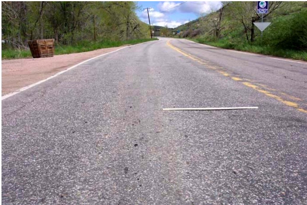
Figure 18: Low Severity Rutting source: (Federal Highway Administration, 2006-2009)
