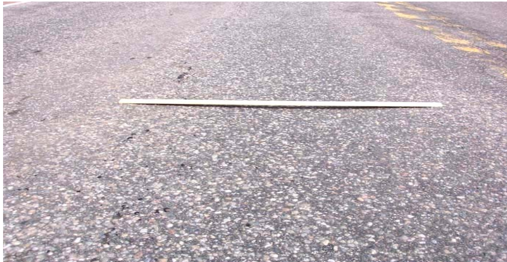
Figure 19: Medium Severity Rutting Source: (Federal Highway Administration, 2006-2009)
