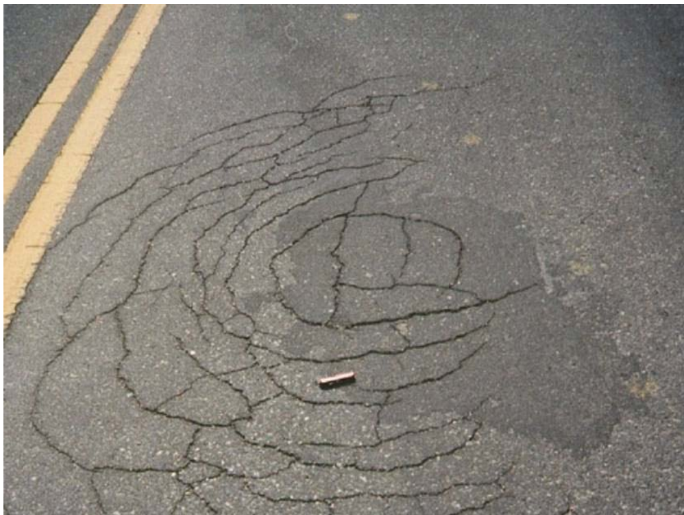
Figure 8: Medium Severity Alligator Cracking Source: (Opus Consultants International (Canada) Limited, 2009)
