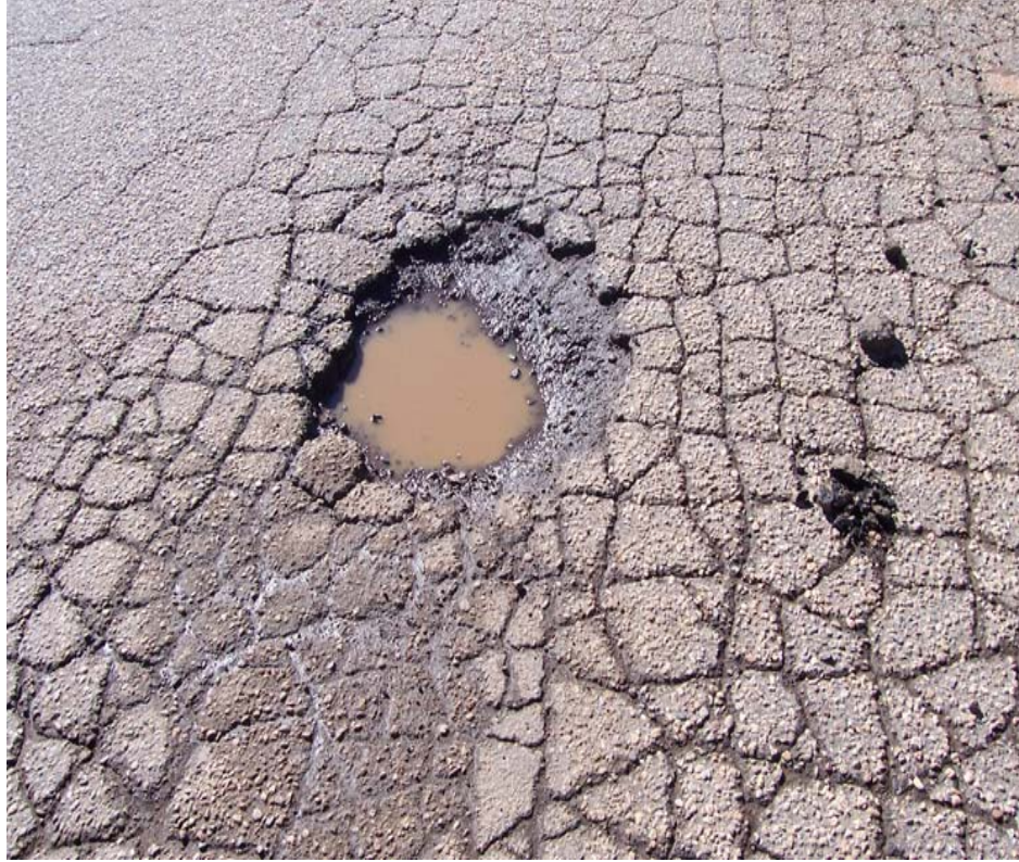
Figure 6: Pothole Surrounded by Alligator Cracking source: (Federal Highway Administration, 2006-2009)
