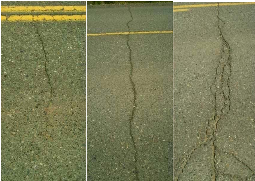
Figure 14: Low, Medium, High Severity Transverse Cracking From Left to Right Respectively
