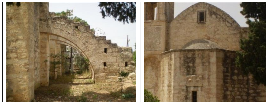
Figure 4.69. Limnia, St. George Church, c.19 th Century. i. Flying Buttresses on the Northern Façade. ii. Semi-Dome over the Apse on the Eastern Façade (©G. Pirlanta).
