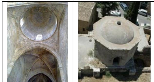
Figure 4.10. Nicosia, St. Nicholas Church, c.5 th Century. i. Gothic Style Ribbed Vaults and Byzantine Dome Structure (©N. Yıldız). ii. Dome before the Renovation (URL 11).
