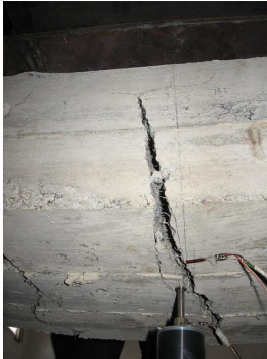
Figure 42: Crack section (2%SP - 1%Fiber)
