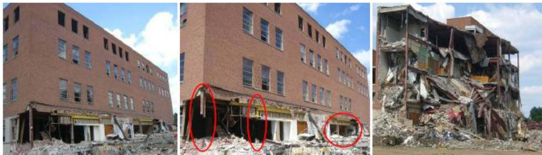
Figure 6: Before and after removal of four first-story columns of the Ohio Union building and its subsequent demolition.
