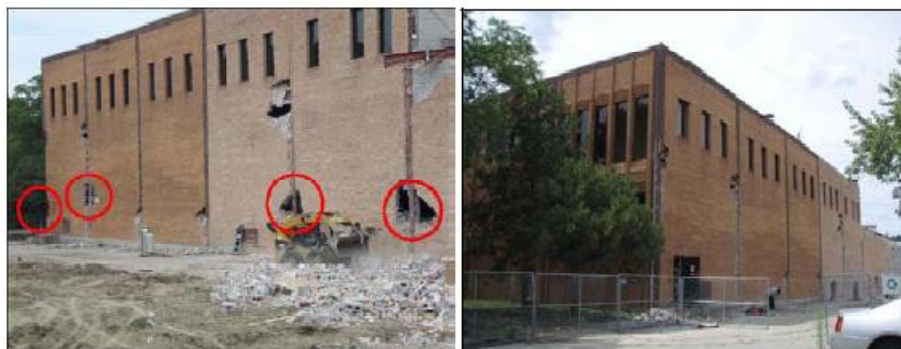
Figure 7: Before and after removal of four first-story columns of the north side of the Bankers Life and Casualty Company building.
