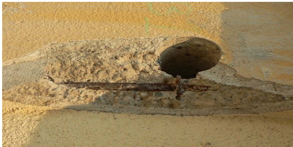
Figure 3-6 Determination of reinforcement bars in column and beam section by removed concrete cover
