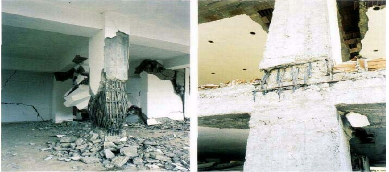
Figure 2-5 Fracture of column, and insufficient reinforcement details in column-beam connection region [Çizmecioğlu, 2007]
