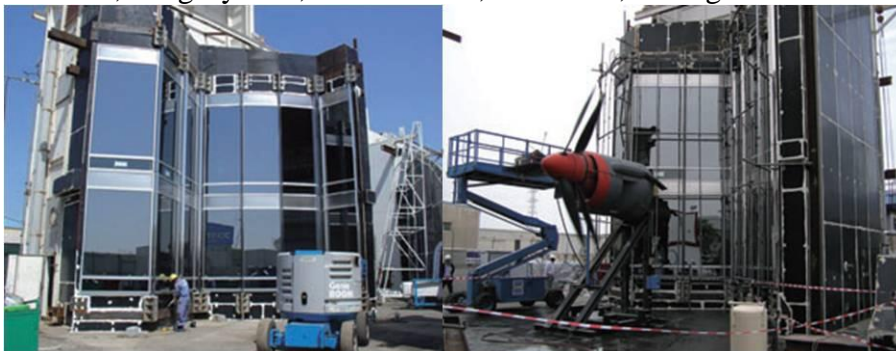
Picture 13: Typical Panel Unit Installation to Building Skeleton (Peter. A. W, Gregory L. S, Mohamed. S, Skidmore, Owings & Merrill. 2007)
