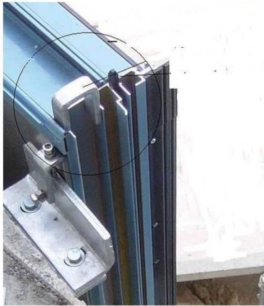
Picture 27: The detail fixing of unitized curtain wall for Al-Jawhara tower (iku® intelligente Fenstersysteme AG. 2008).
