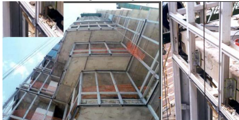
Picture 5: Installation of Mullion and Transoms for the Glass Fixing (Wong W.M. R)
