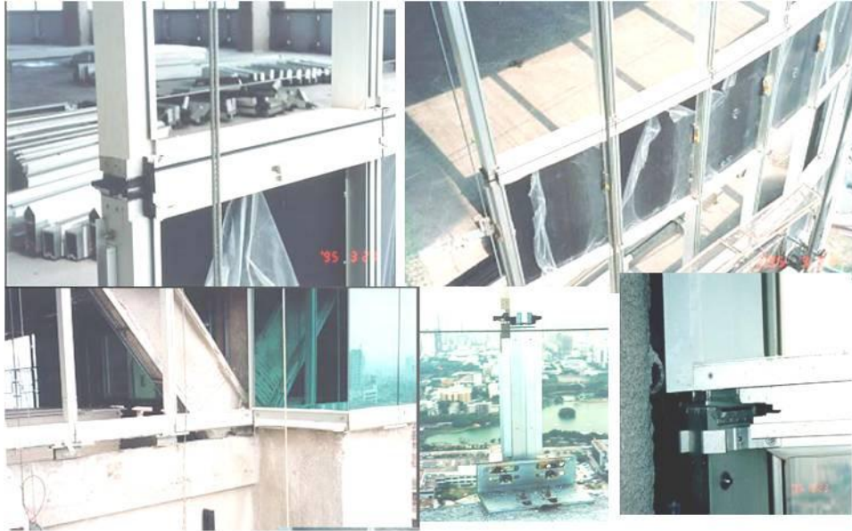
Picture 7: Anchorage Installations for Mullions and Transoms and Glass Panes with Bracket for Shun Hing Plaza Tower (Wong W.M.R)
