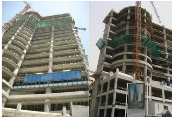
Picture 10: The Erection of Unitized Curtain Wall on Building Skeleton for Al-Jawhara Tower, Kuwait. http://www.iku-windows.com/recent_news/fortschritt
