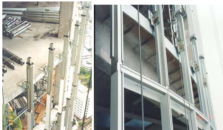
Picture 25: The Installed Mullions and Transoms for the Stick Curtain Wall in Shun Hing Plaza (Wong, W. M. R)
