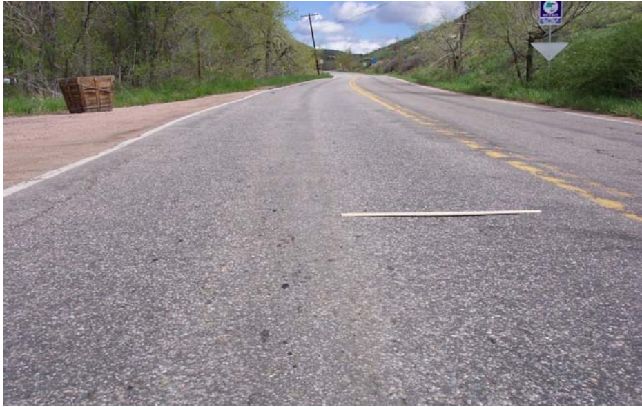
Figure 24: Low Severity Rutting (Federal Highway Administration, 2006-2009, p. 16)
