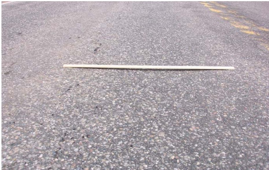
Figure 25: Medium Severity Rutting (Federal Highway Administration, 2006-2009, p. 15)
