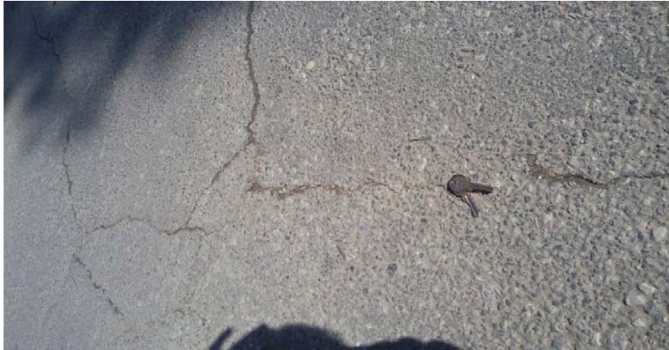
Figure 61: Alligator Cracking, Low Severity
