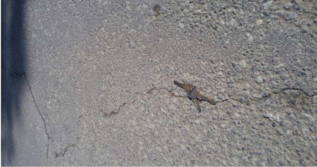
Figure 55: Transverse, Medium Severity
