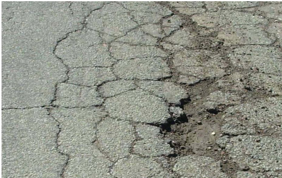
Figure 15: Low Severity Pothole (Opus Consultants International (Canada) Limited, 2009, p. 49)
