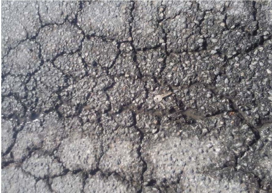
Figure 59: Alligator Cracking, High Severity
