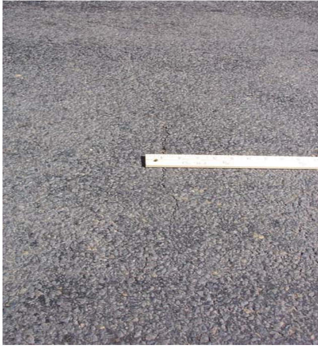
Figure 12: Low Severity Transverse Cracking (Federal Highway Administration, 2006-2009, p. 10)
