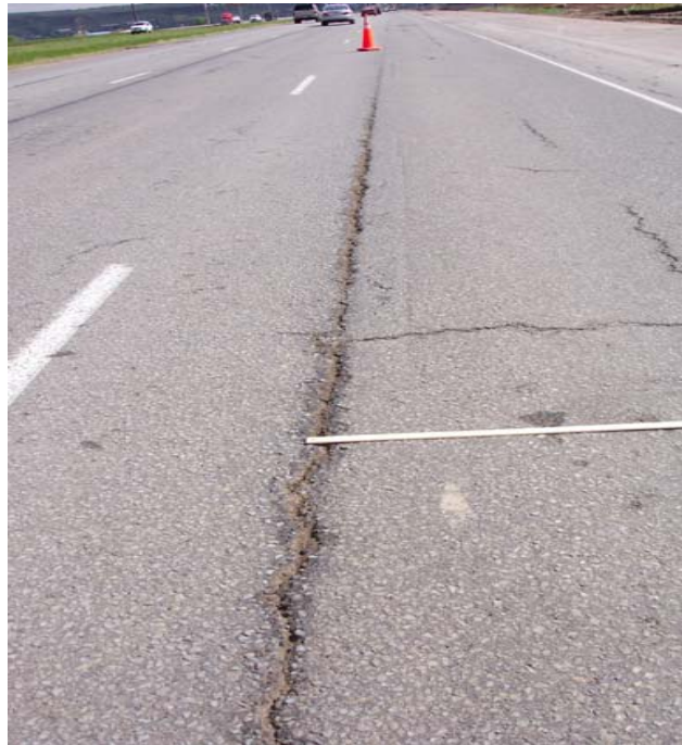
Figure 11: High Severity Longitudinal Cracking (Federal Highway Administration, 2006-2009, p. 7)
