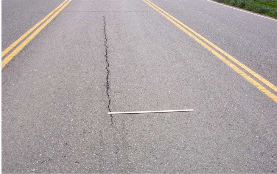
Figure 10: Medium Severity Longitudinal Cracking (Federal Highway Administration, 2006-2009, p. 8)
