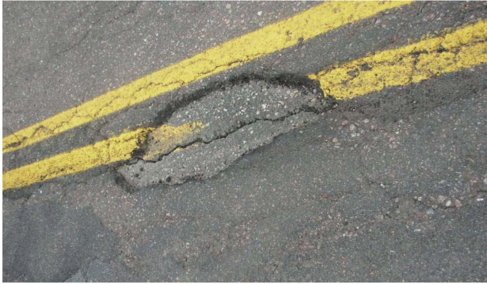
Figure 16: Moderate Severity Pothole (Opus Consultants International (Canada) Limited, 2009, p. 49)
