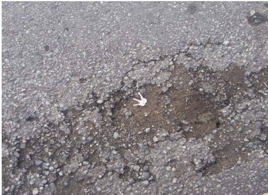
Figure 58: Potholes, Medium Severity
