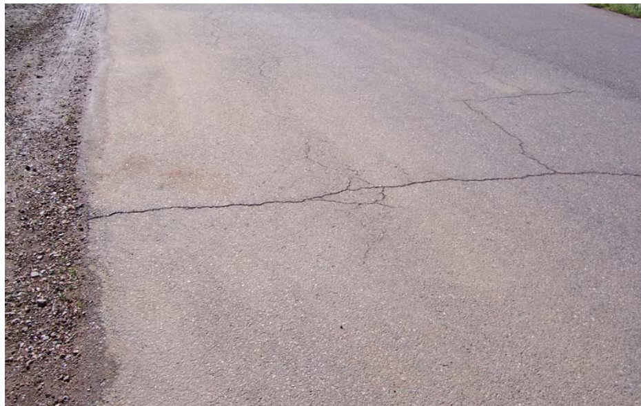
Figure 13: Medium Severity Transverse Cracking (Federal Highway Administration, 2006-2009, p. 10)
