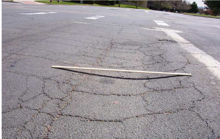
Figure 26: High Severity Rutting (Federal Highway Administration, 2006-2009, p. 15)
