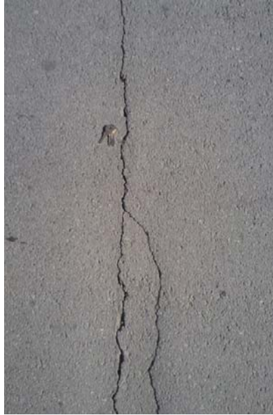
Figure 51: Longitudinal, High Severity
