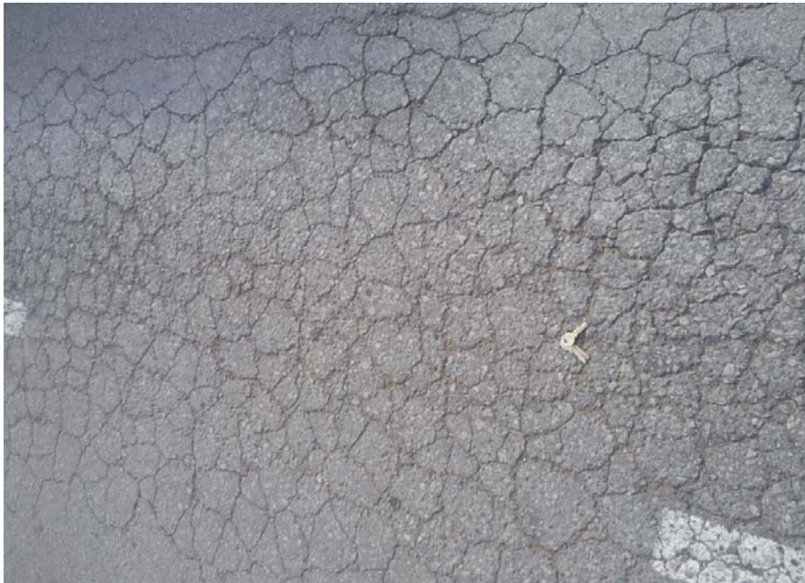
Figure 60: Alligator Cracking, Medium Severity
