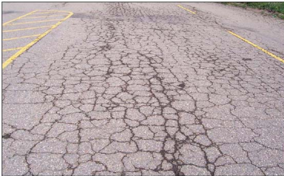
Figure 8: High Severity Alligator Cracking (Federal Highway Administration, 2006-2009, p. 5)
