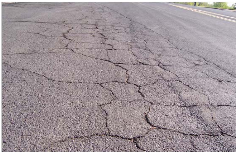
Figure 7: Medium Severity Alligator Cracking (Federal Highway Administration, 2006-2009, p. 6)
