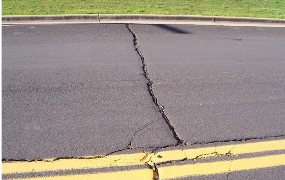
Figure 14: High Severity Transverse Cracking (Federal Highway Administration, 2006-2009, p. 9)
