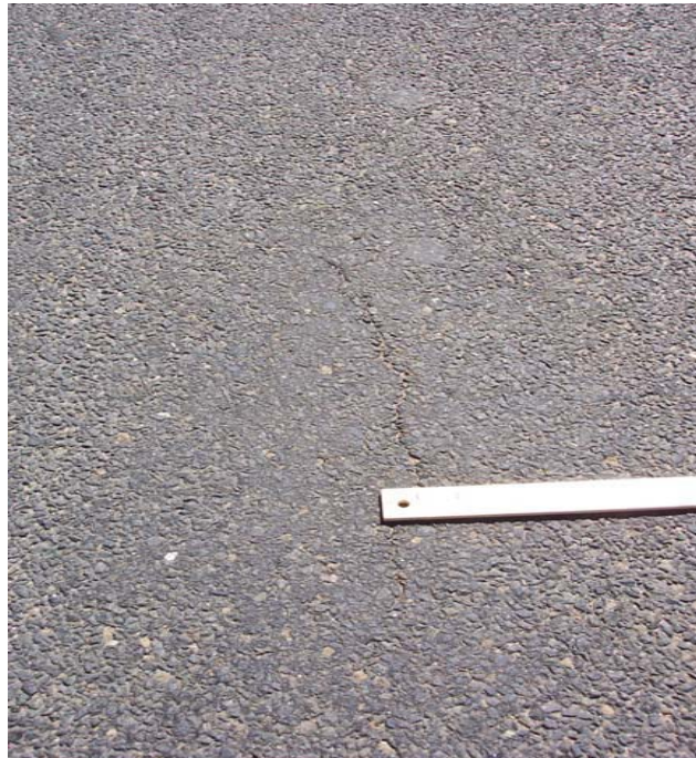
Figure 9: Low Severity Longitudinal Cracking (Federal Highway Administration, 2006-2009, p. 8)
