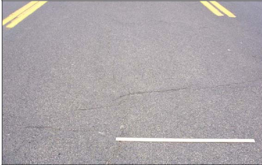
Figure 6: Low Severity Alligator Cracking (Federal Highway Administration, 2006-2009, p. 6)
