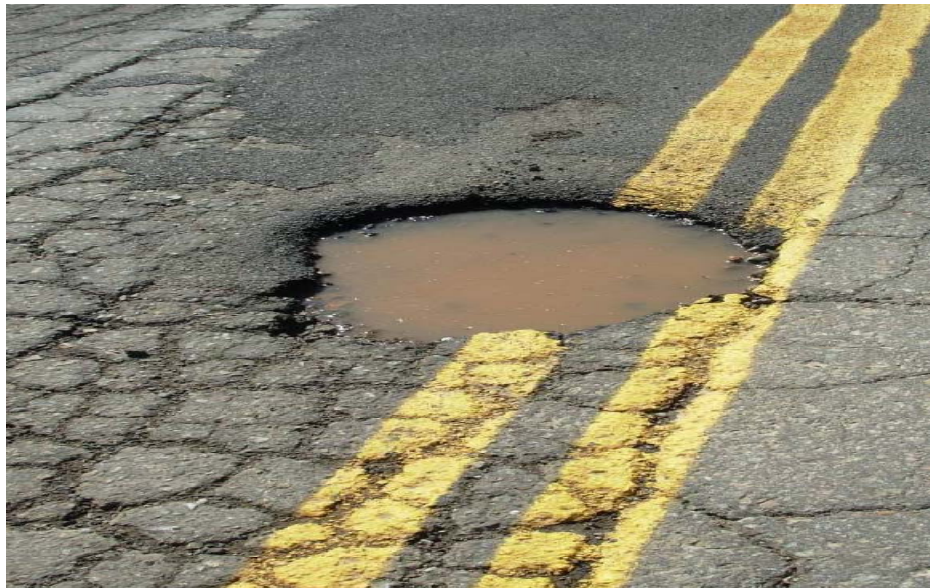
Figure 17: High Severity Pothole (Opus Consultants International (Canada) Limited, 2009, p. 50)
