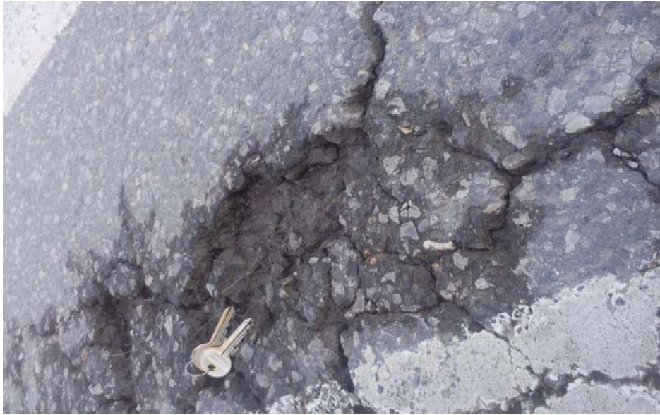
Figure 57: Potholes, High Severity
