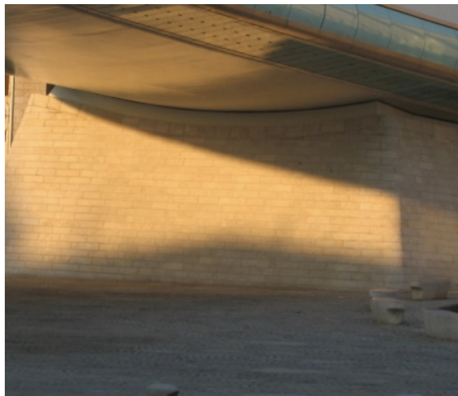
Figure 35. The pedestrian over cross, resting on bases covered with stone, taken from below the Bridge of Strings (Calatrava, 2011).
