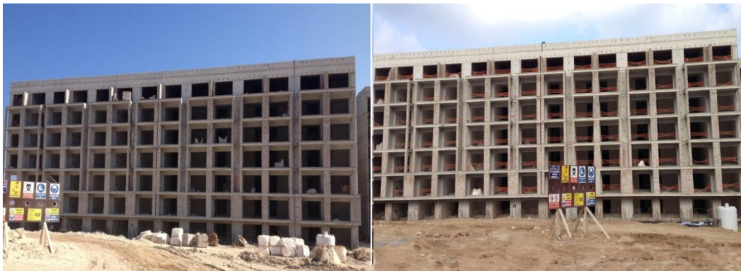
Figure 5.9. Safety net system in LPH project (2)
