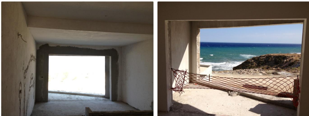
Figure 5.8. Safety net system in LPH project (1)
