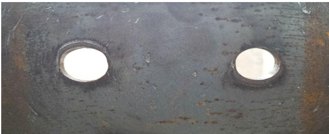
Figure 4.16. W200x200 connection deformation
