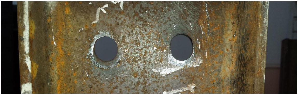
Figure 4.20. W160x160 Connection deformation
