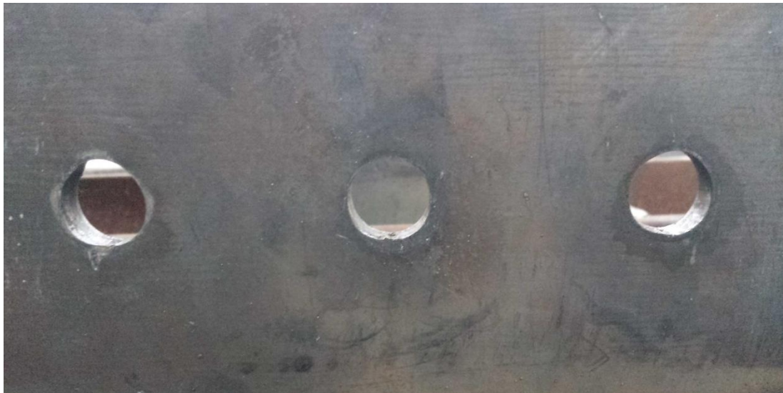
Figure 4.14. W300x200 Connection deformation as enlargement of bolt holes
