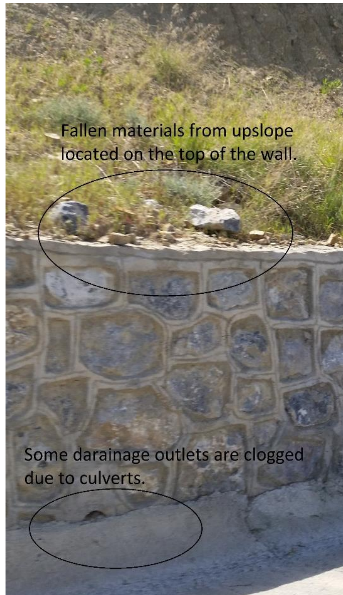
Figure B.4. Clogged drainage outlets.
