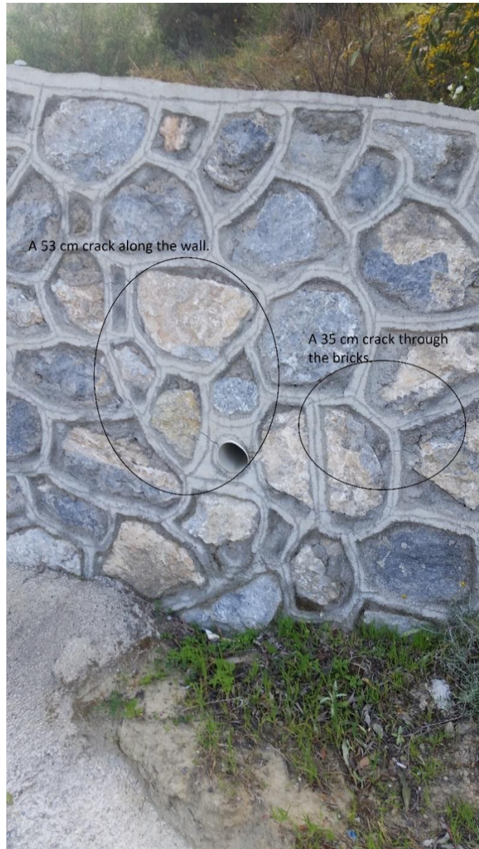
Figure B.3. Site 10-cracks along the wall.
