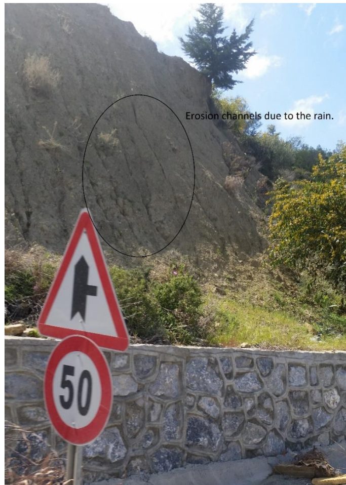
Figure B.5. Erosion channels in the backfill soil.
