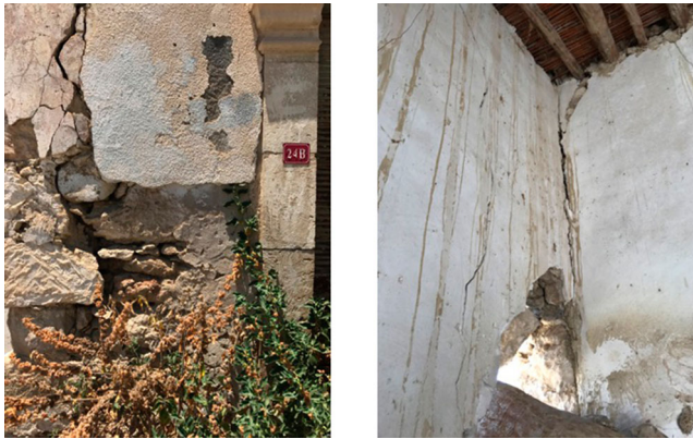
Figure 10. A vertical and a diagonal crack in the walls of Büyükkonuk1 olive mill.
