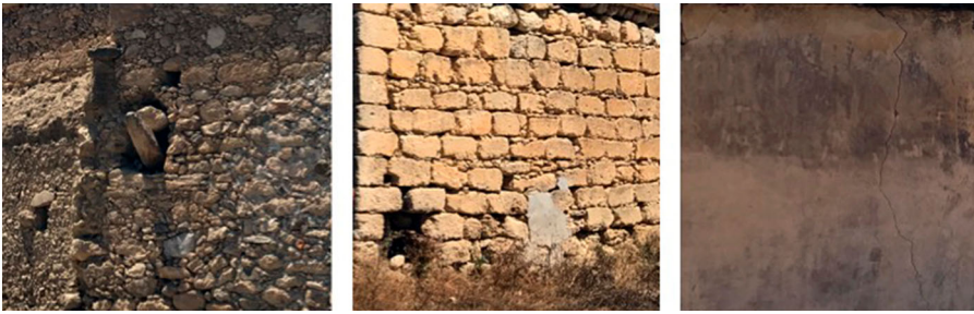
Figure 12. (a) A collapsed part in the walls of the Büyükkonuk 1 mill, (b) a large vertical crack in a wall of the Boltaşlı mill, and (c) a large diagonal crack in a wall of the Taşlıca mill.
