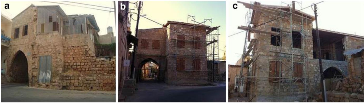
Fig. 6. The state of the building before restoration (a) and after restoration (b, c) (Photos by .....)
