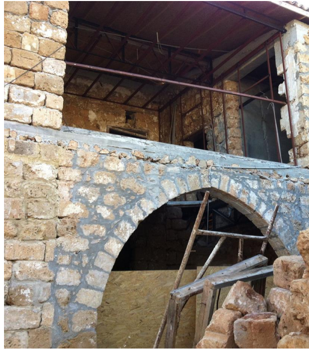
Fig. 7. The uses of concrete beams and cement mortar for the restoration work (Photo by .....)
