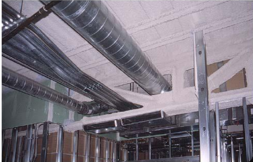
Figure 1.4: STMF with piping and ductwork [4]
