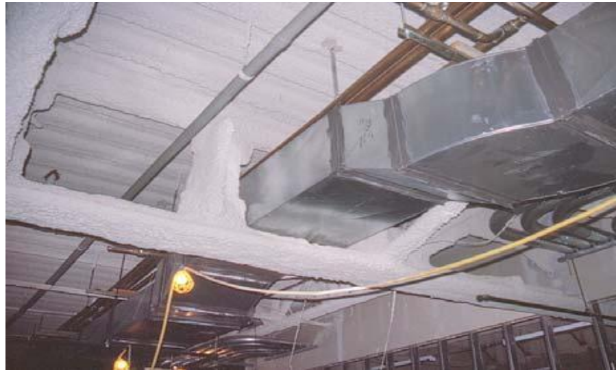
Figure 1.5: STMF with piping and ductwork [4]
