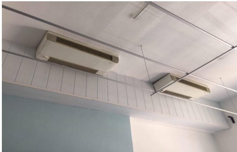
Figure 20: Air conditioning of A18 Classroom (Taken by author)
