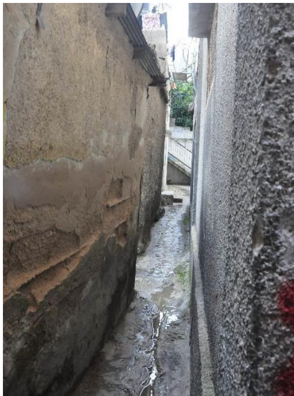
Figure 23: Water leakage and swamp in the alley
